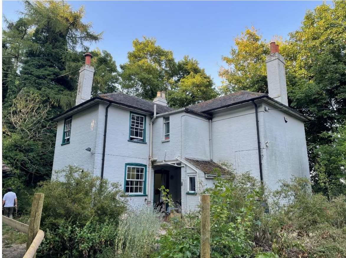
Figure 7 The rear of the house showing the modern infill structures and proliferation of modern pipework.
