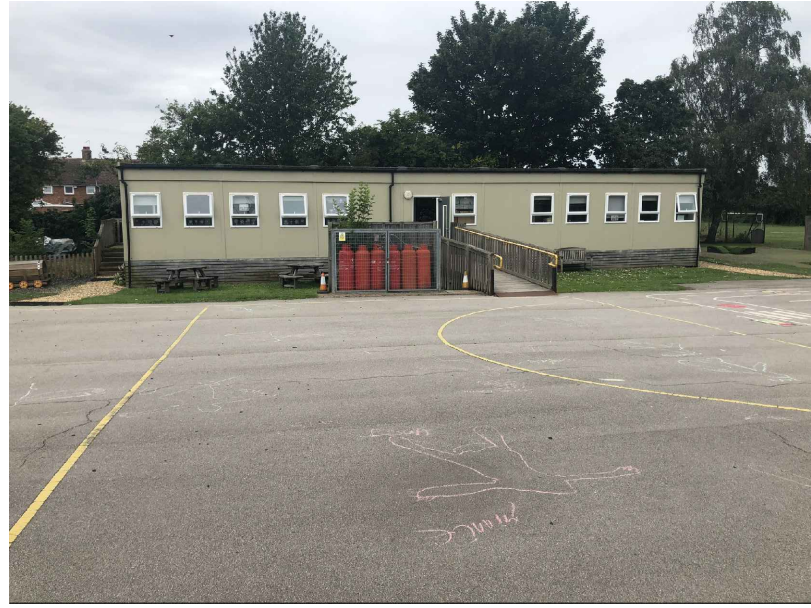
Survey photo of the existing mobile Front elevation to existing school hard play
