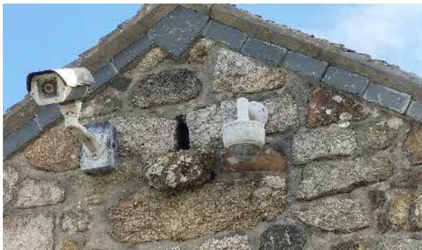
Figure 3. The small hole at the western gable apex
