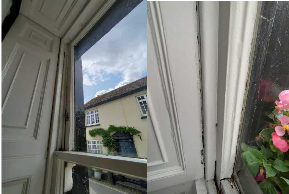
Figure 10 – Details of poor state of repair of Dining Room and Sitting Room windows (Ground Floor)
