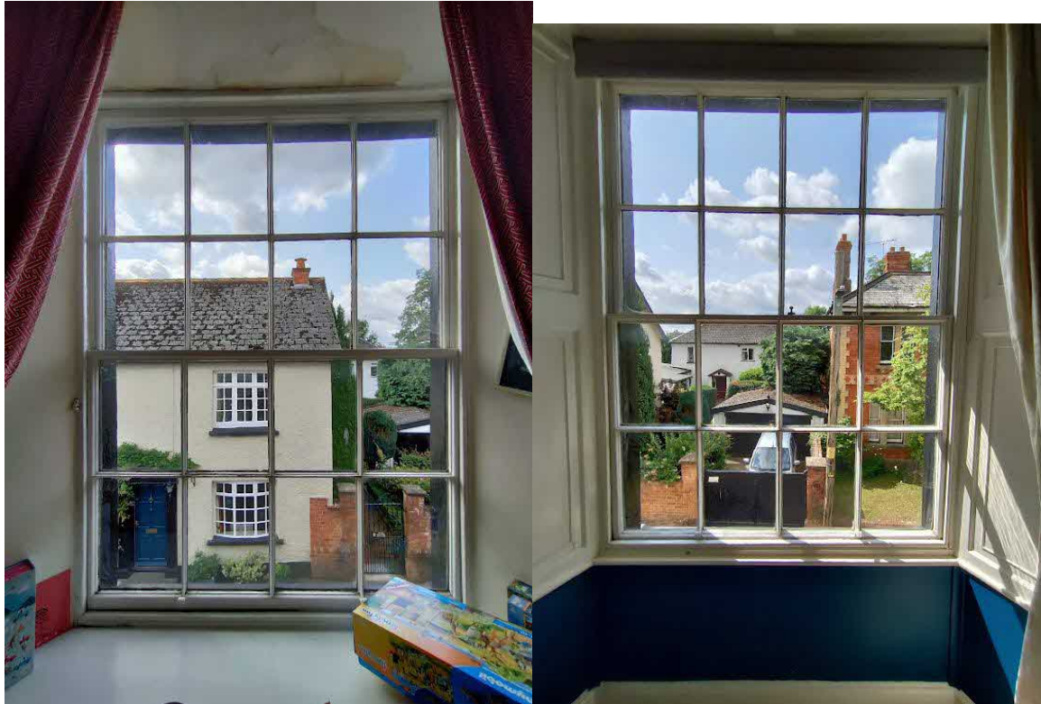
Figure 13 – The new Ground Floor windows would match the original 8 over 8 pane windows in Bedroom 2 and Bedroom 3 (First Floor)
