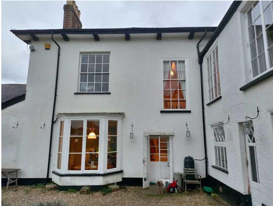
Figure 6 – View of rear elevation showing Ground Floor Kitchen bay window and Second Floor original sash windows on stairwell and Dressing Room, with side view of rear extension windows on the right (all unaffected by the proposals)
