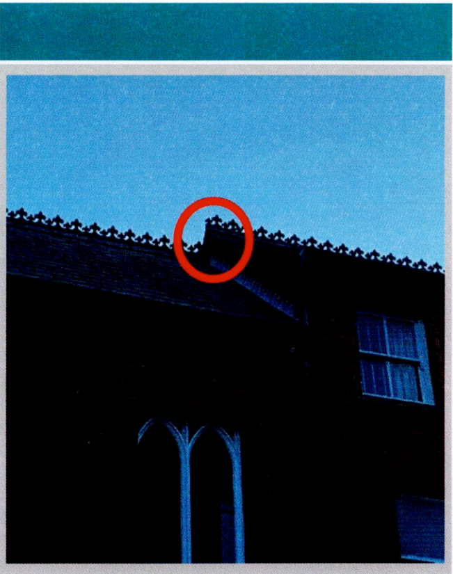
Photograph 2: Roost 1, a common pipistrelle day roost (1 x bat) beneath a roof tile in a section of B1 that is being retained
