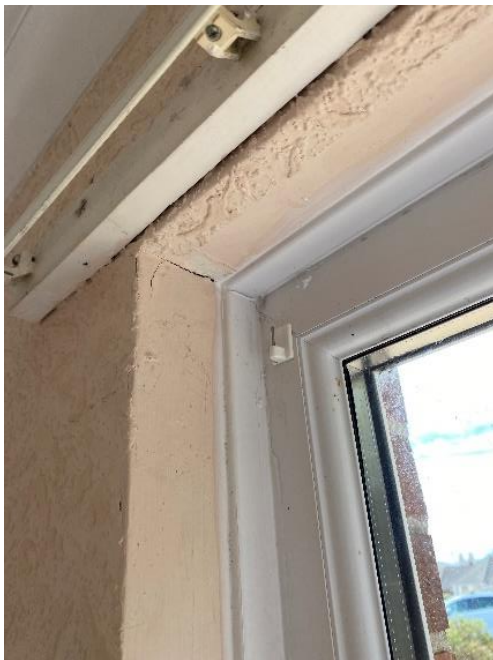
Photo 55: Crack at high level to the East side of the window to the front elevation of the Front Bedroom
