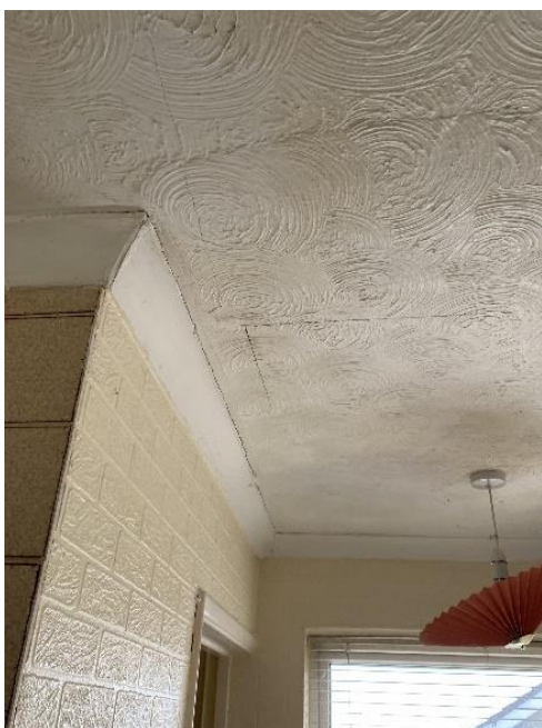
Photo 75: Cracking to the Kitchen ceiling within the extension
