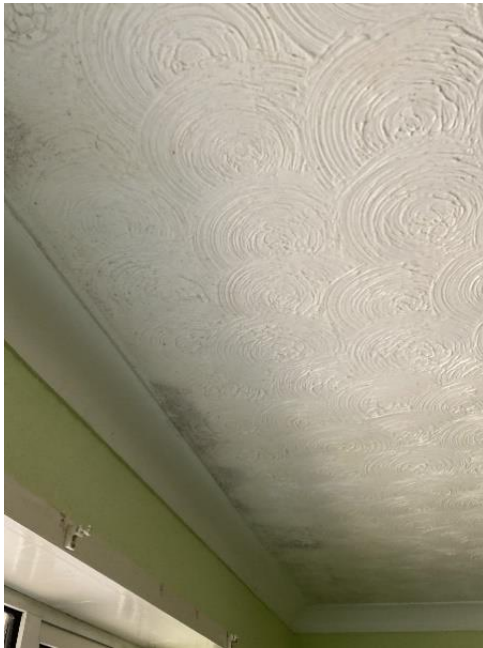
Photo 71: Damp staining to the ceiling
