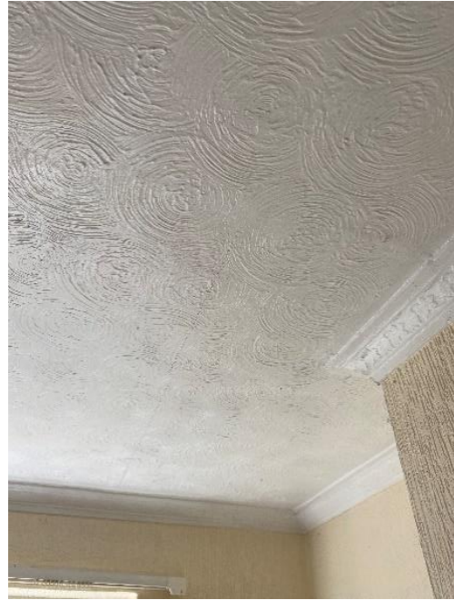
Photo 66: Cracking to the Rear Reception Room ceiling
