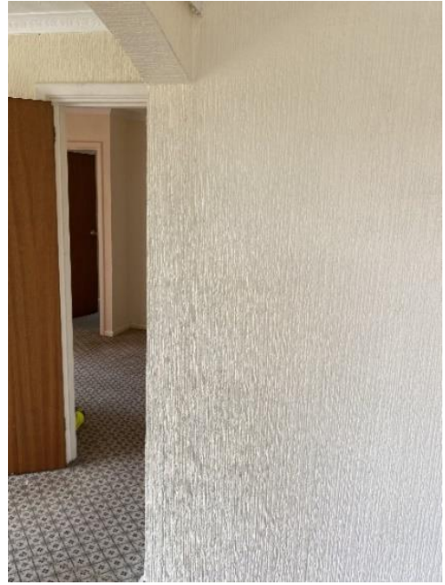
Photo 68: Tapered vertical crack to the reveal to the side of the opening within the wall which separates the Reception Rooms
