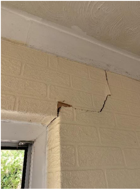
Photo 77: Stepped crack above the back door to the Kitchen
