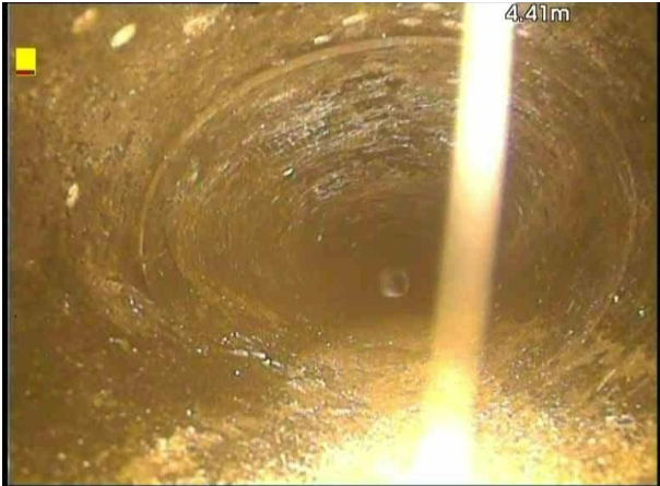
Sec_5_Insp_1_MH3X_36059.jpg, 00:01:28, 4.41 m Deformed sewer or drain, 30%
