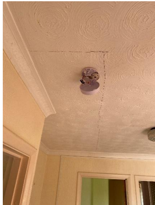
Photo 58: Cracking to the ceiling above the Entrance
