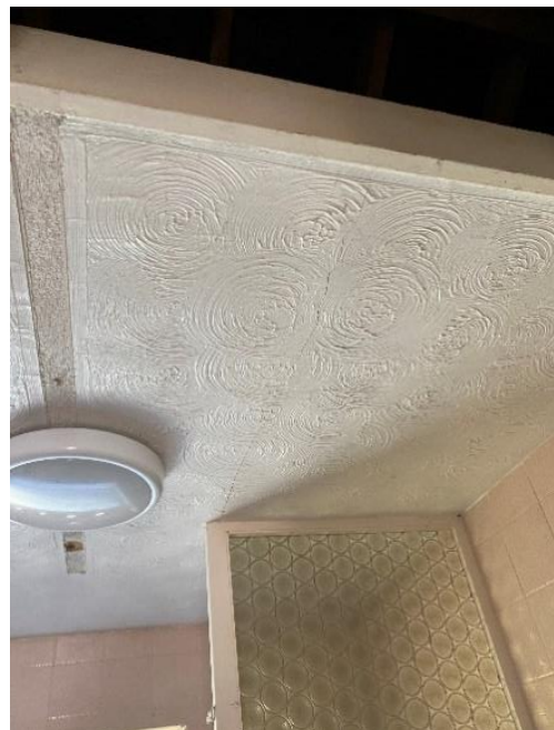
Photo 60: Cracking to the Bathroom ceiling
