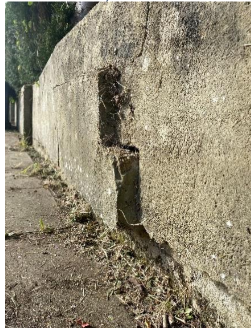
Photo 52: Cracking and movement to the boundary wall to the left-hand side of the property. Damage at location of Cherry tree
