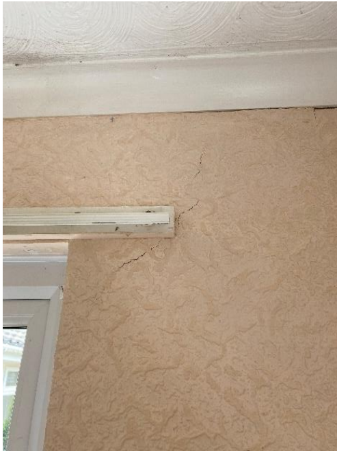
Photo 53: Isolated diagonal crack above the South side of the window to the side elevation of the Front Bedroom
