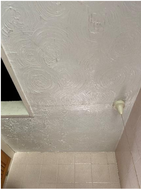
Photo 61: Cracking to the Bathroom ceiling
