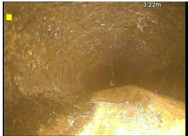
Sec_5_Insp_1_MH3X_38867.jpg, 00:01:08, 3.22 m Deformed sewer or drain, 15%
