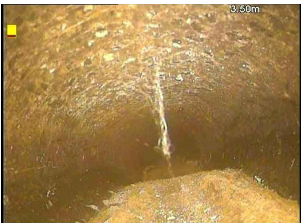
Sec_5_Insp_1_MH3X_19791.jpg, 00:01:15, 3.50 m Deformed sewer or drain, 25%
