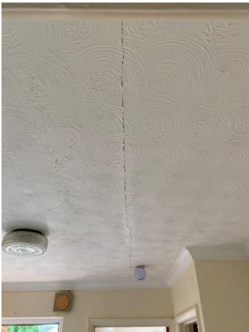
Photo 59: Cracking to the Entrance Hall ceiling
