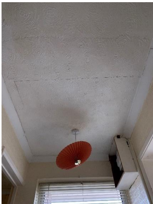
Photo 73: Cracking to the Kitchen ceiling within the extension
