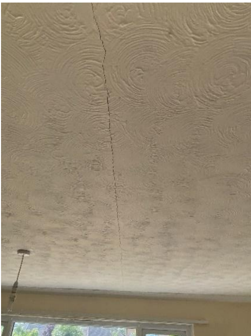
Photo 63: Cracking to the Front Reception Room ceiling
