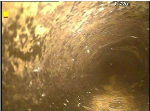
Sec_5_Insp_1_MH3X_29315.jpg, 00:00:26, 0.72 m Deformed sewer or drain, 20%
