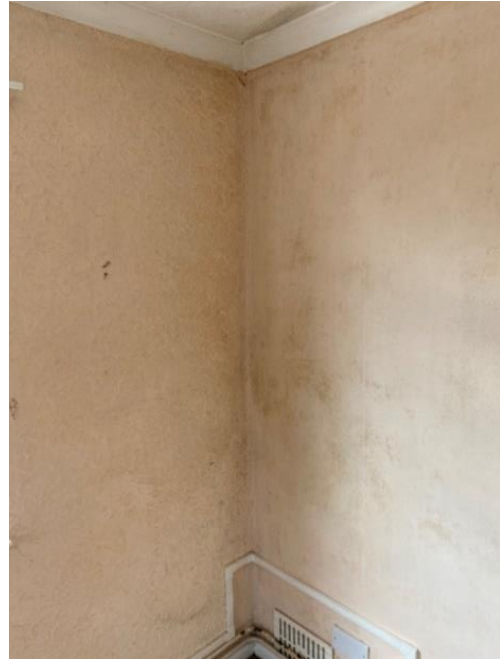
Photo 70: Damp staining to the external walls
