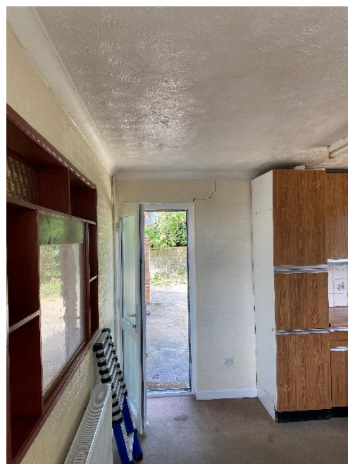
Photo 76: Stepped crack above the back door to the Kitchen
