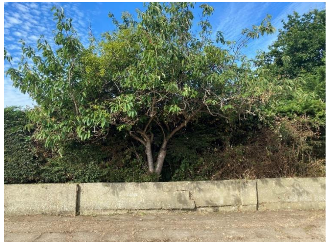
Photo 48: Cracking and movement to the boundary wall to the left hand side of the property
