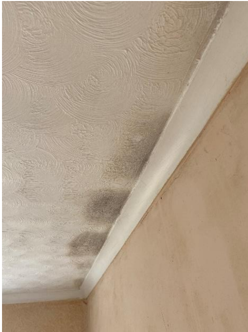
Photo 69: Damp staining to the ceiling
