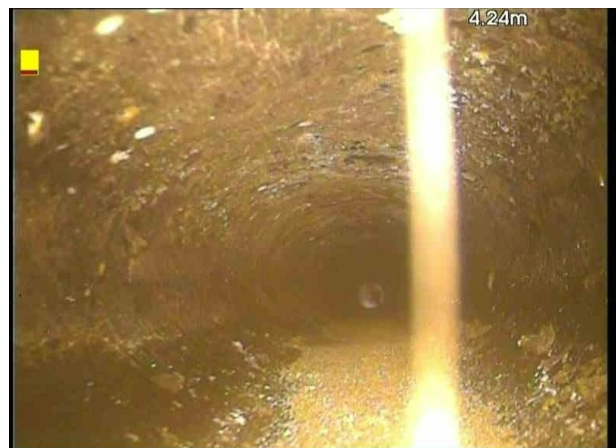
Sec_5_Insp_1_MH3X_38101.jpg, 00:01:26, 4.24 m Deformed sewer or drain, 20%
