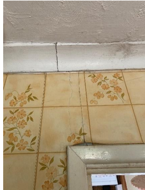
Photo 84: Cracking above the Kitchen door within the Shower Room
