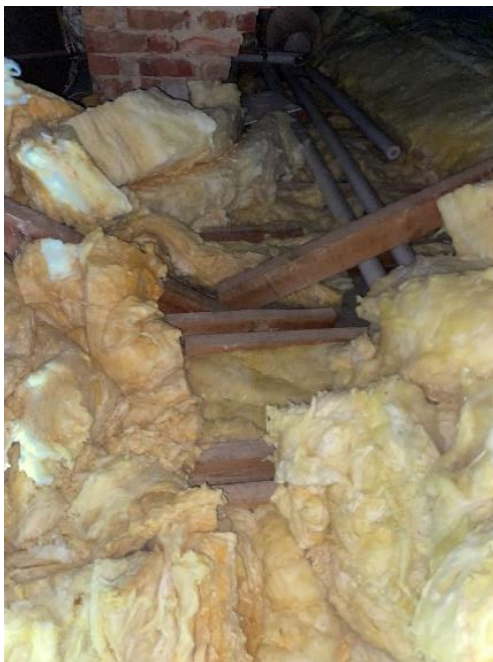
Photo 91: The ceiling joists are not fixed together where they were spliced over the central spine wall
