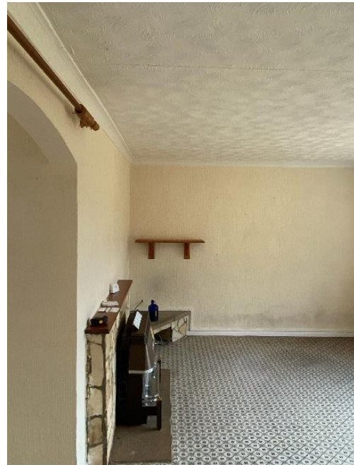
Photo 72: Damp staining at low level to the external walls
