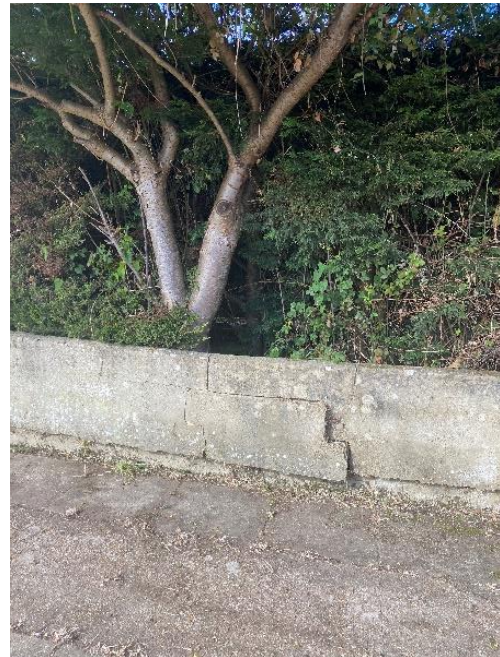
Photo 50: Cracking and movement to the boundary wall to the left hand side of the property. Damage at location of Cherry tree
