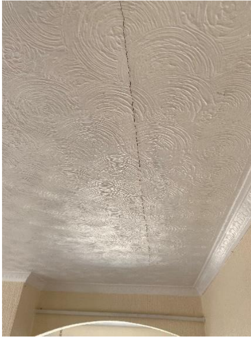
Photo 65: Cracking to the Rear Reception Room ceiling
