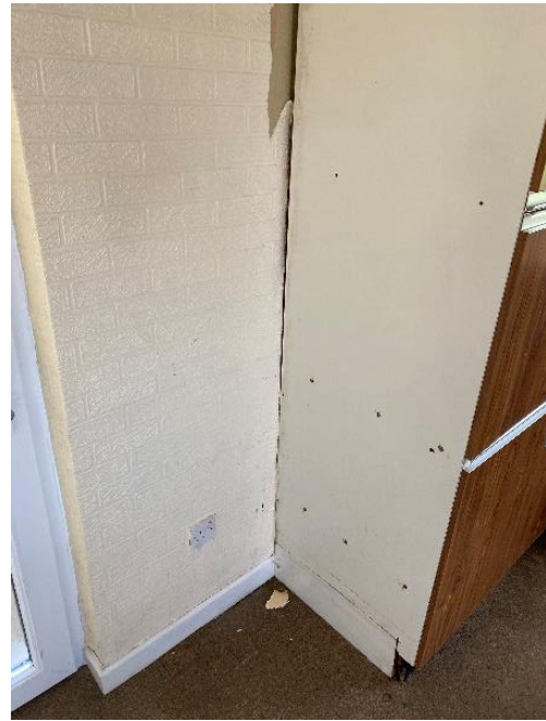
Photo 78: Movement to the external wall to the side of the back door to the Kitchen
