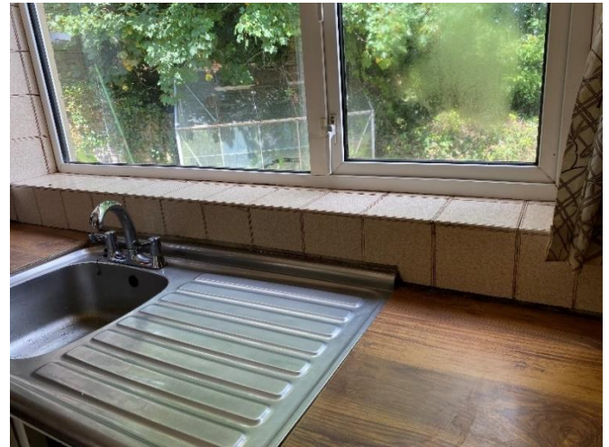
Photo 82: Gap between the top of the worktops and the wall tiles above to the rear external wall of the Kitchen
