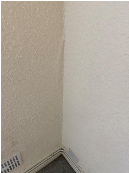
Photo 57: Stressing to the wallpaper at the junction between the Rear Bedroom wall and the external wall within the Middle Bedroom
