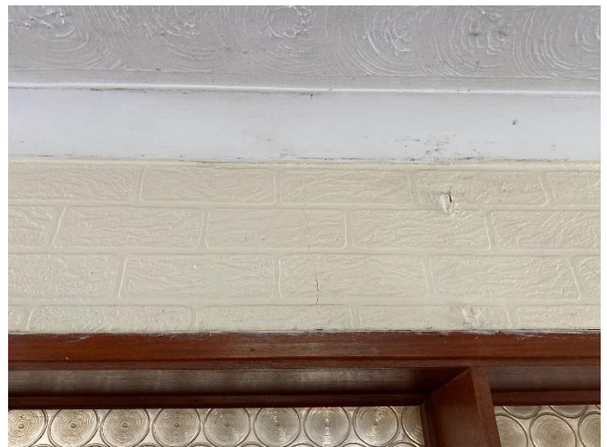
Photo 80: Hairline crack at high level to the rear external elevation of the main property within the Kitchen
