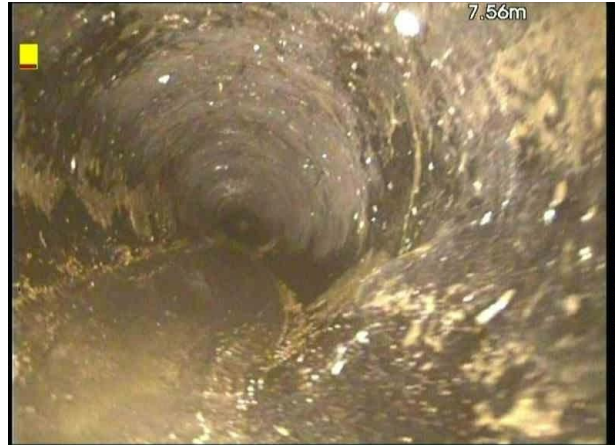
Sec_7_Insp_1_MH4X_15154.jpg, 00:01:37, 7.56 m Deformed sewer or drain, 10%
