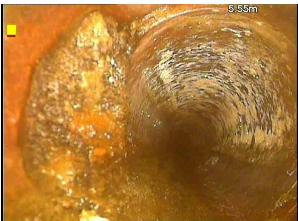
Sec_8_Insp_1_MH5X_30211.jpg, 00:01:09, 5.55 m Attached deposits, encrustation at joint from 7 o'clock to 11 o'clock, 15% cross-sectional area loss
