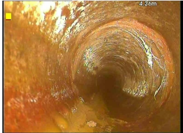
Sec_8_Insp_1_MH5X_65006.jpg, 00:00:57, 4.36 m Joint displaced, medium
