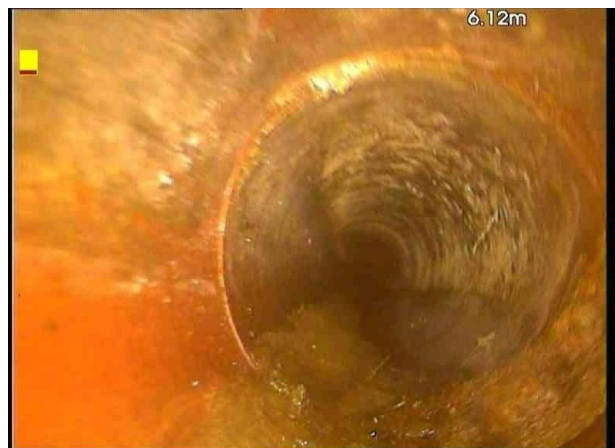
Sec_8_Insp_1_MH5X_36643.jpg, 00:01:14, 6.12 m Attached deposits, encrustation at joint from 4 o'clock to 6 o'clock, 5% cross-sectional area loss
