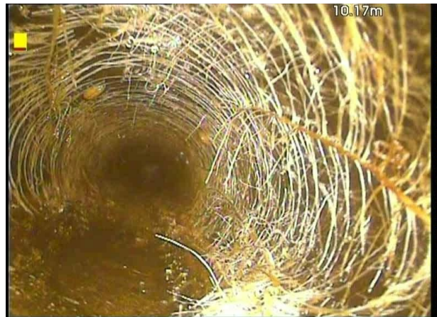
Sec_7_Insp_1_MH4X_42678.jpg, 00:02:13, 10.17 m Roots, fine, start
