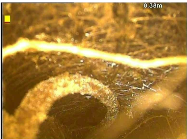
Sec_9_Insp_1_UnknownX_23973.jpg, 00:00:23, 0.38 m Roots, tap
