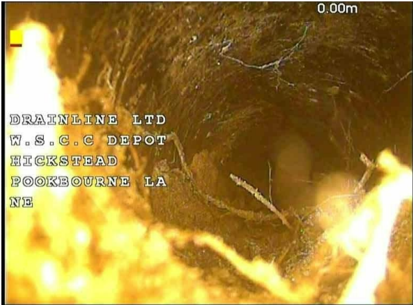
Sec_9_Insp_1_UnknownX_57778.jpg, 00:00:03, 0.10 m Settled deposits, fine, 15% cross-sectional area loss
