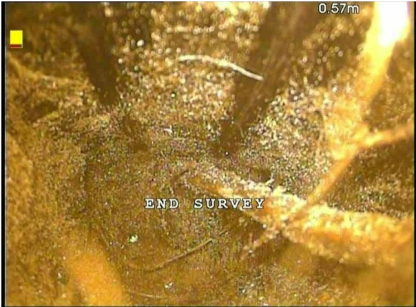
Sec_9_Insp_1_UnknownX_35906.jpg, 00:00:54, 0.57 m Settled deposits, fine, 100% cross-sectional area loss
