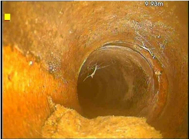
Sec_8_Insp_1_MH5X_3755.jpg, 00:01:59, 9.93 m Settled deposits, coarse, 15% cross-sectional area loss
