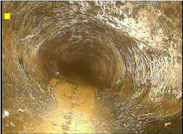
Sec_7_Insp_1_MH4X_9366.jpg, 00:00:23, 0.00 m Deformed sewer or drain, 20%, start
