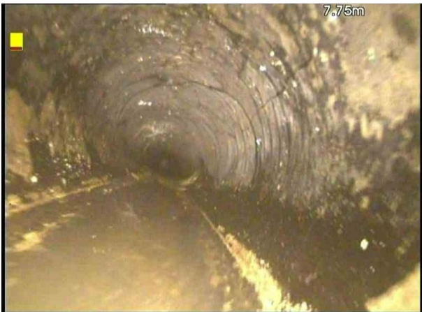
Sec_7_Insp_1_MH4X_42728.jpg, 00:01:59, 9.38 m Deformed sewer or drain, 15%
