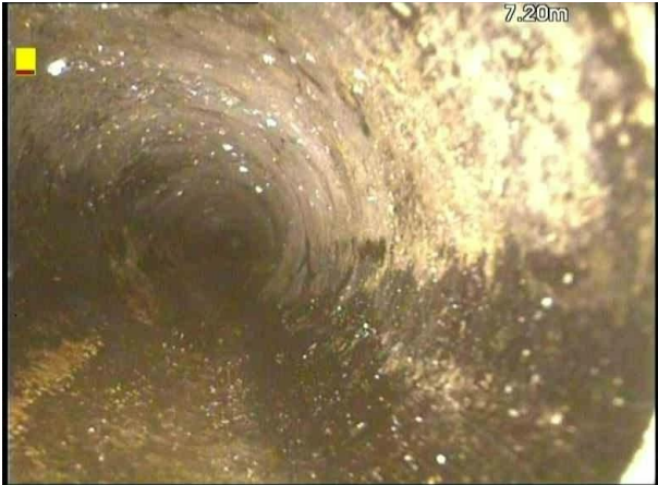
Sec_7_Insp_1_MH4X_820.jpg, 00:01:33, 7.20 m Deformed sewer or drain, 10%
