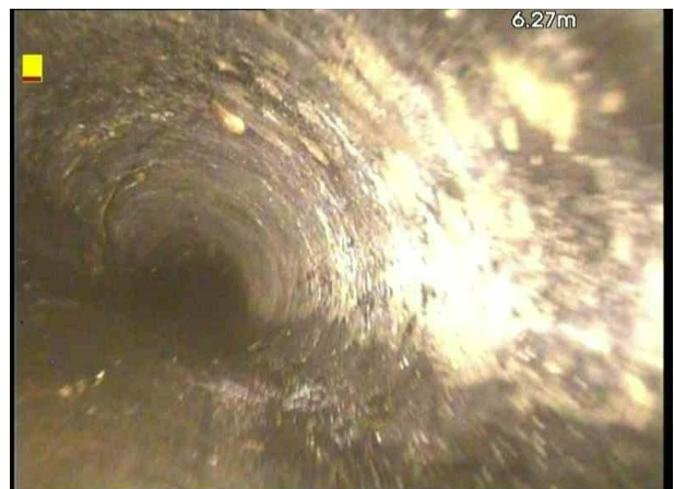
Sec_7_Insp_1_MH4X_20830.jpg, 00:01:23, 6.27 m Deformed sewer or drain, 15%
