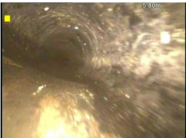
Sec_7_Insp_1_MH4X_46663.jpg, 00:01:20, 5.80 m Deformed sewer or drain, 15%
