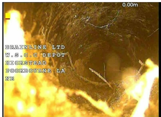
Sec_9_Insp_1_UnknownX_3424.jpg, 00:00:23, 0.38 m Settled deposits, fine, 30% cross-sectional area loss
