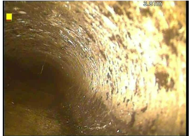
Sec_7_Insp_1_MH4X_36190.jpg, 00:01:05, 3.81 m Deformed sewer or drain, 30%, start
