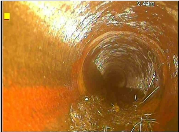
Sec_8_Insp_1_MH5X_57050.jpg, 00:00:41, 2.44 m Roots, fine at joint
