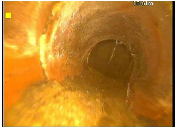
Sec_8_Insp_1_MH5X_62410.jpg, 00:02:07, 10.61 m Attached deposits, encrustation from 5 o'clock to 8 o'clock, 10% cross-sectional area loss
