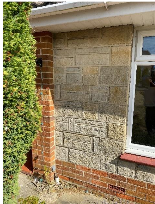
Photo 4: Cracking to the stonework to the front elevation of the Reception Room
