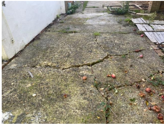
Photo 8: Appeared to have been widening of cracks and further movement to the concrete slab adjacent to the West side elevation of the property – 12th October 2022
