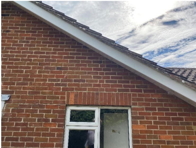
Photo 11: Cracking and repointing to the wall above the Middle Bedroom window
