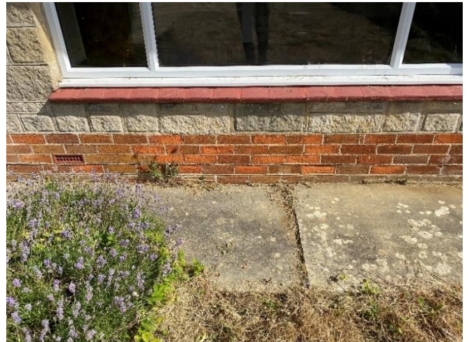
Photo 6: Spalling of brickwork below the Reception Room window
