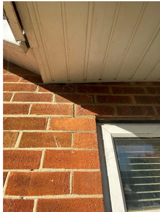
Photo 4: Crack to the wall above the window to the East side elevation of the Kitchen extension. At the junction between the main property and the extension to the rear - 13th October 2022
