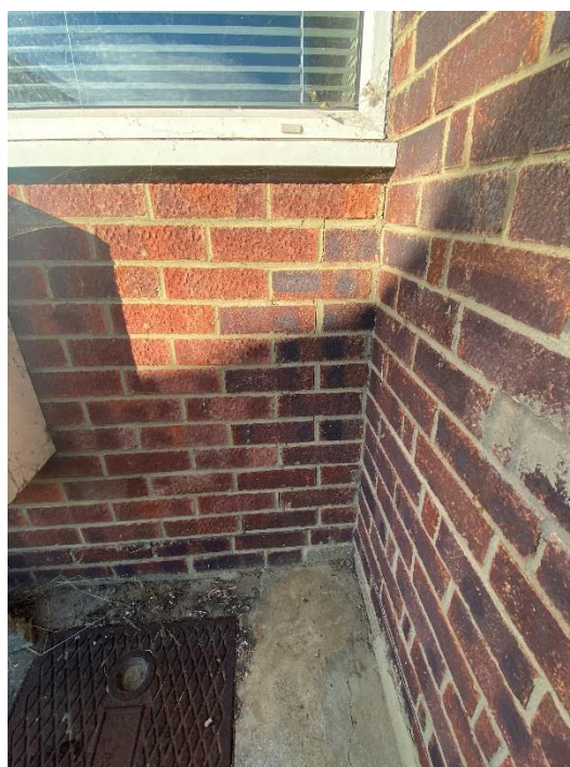
Photo 6: Crack below the window to the East side elevation of the Kitchen - Additional cracking - 12th October 2022
