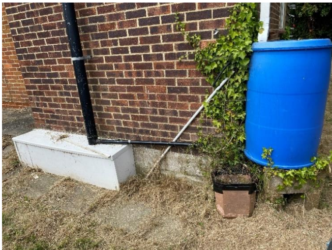
Photo 35: Foul and surface water downpipes and inspection chamber (not shown) adjacent to the East side elevation of the extension
