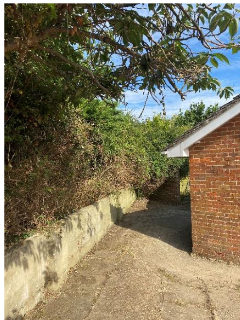
Photo 42: Trees and vegetation adjacent to the left hand side elevation of the property
