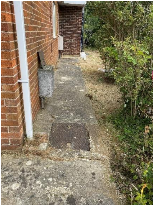
Photo 31: Inspection chambers adjacent to the right hand side elevation of the main property
