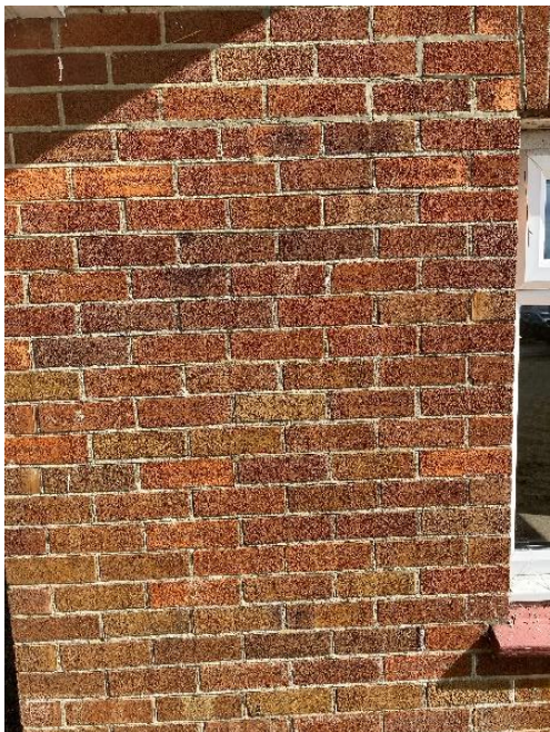
Photo 3: General condition of the brickwork to the external elevations of the property
