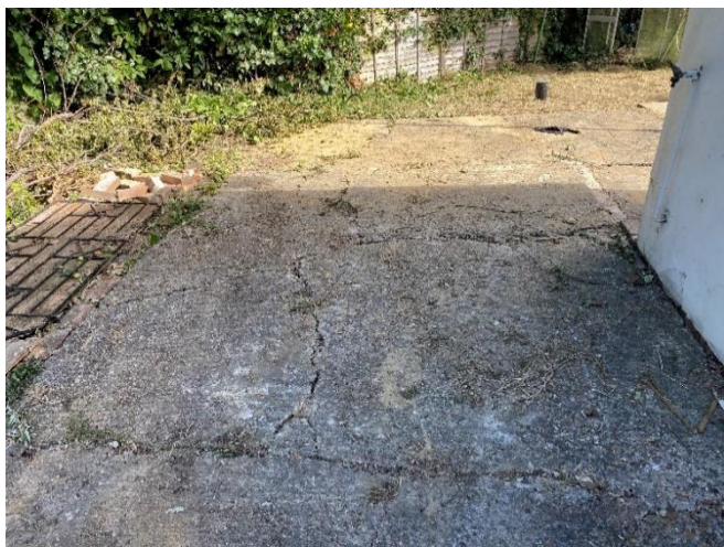
Photo 25: Cracked and dropped concrete slab to the rear of the property. Old garage removed.
