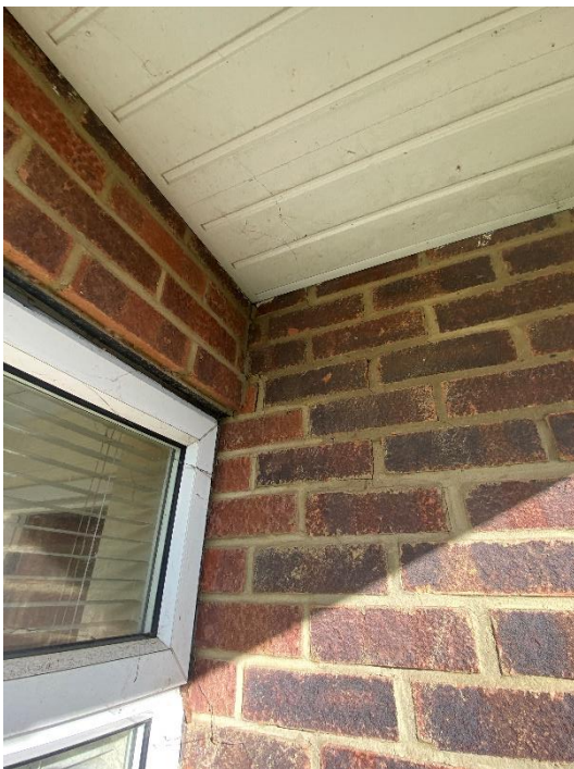
Photo 5: Crack above the window to the East side elevation of the Kitchen - Additional cracking - 12th October 2022
