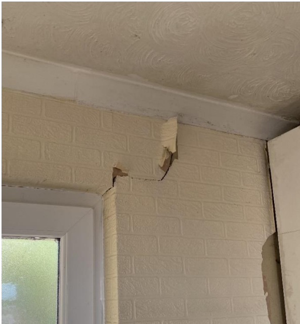
Photo 1: Crack above the back door to the West side elevation of the Kitchen extension - 13th July 2022
