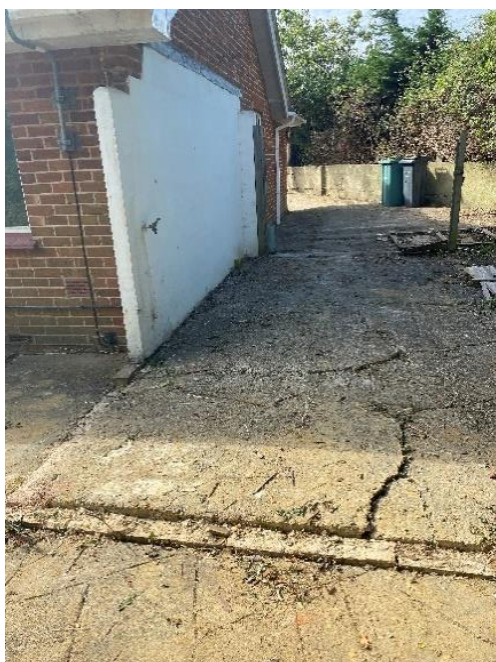
Photo 23: Cracked and dropped concrete slab to the rear of the property. Old garage removed. Surface water was thought to pool on the path against the building
