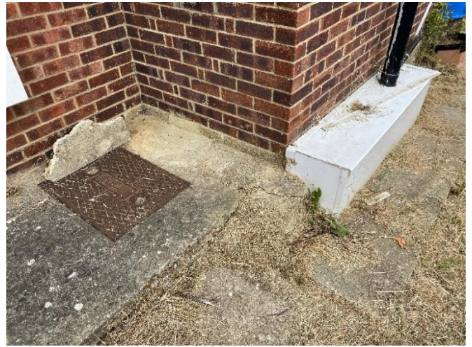
Photo 34: Foul and surface water downpipes to the East side elevation of the extension. Inspection chamber adjacent to the rear right hand corner of the main property
