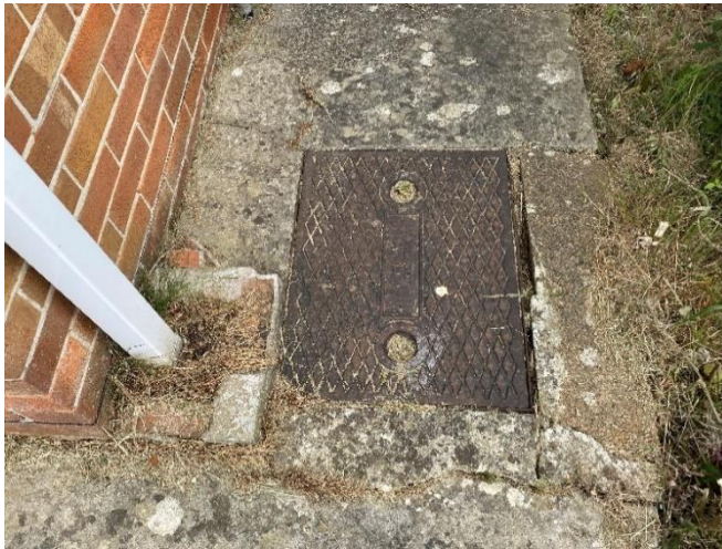
Photo 33: Rainwater gulley and inspection chambers adjacent to the right hand side elevation of the main property
