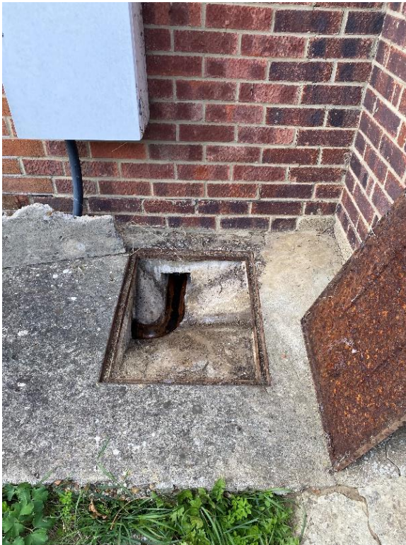
Photo 11: Inspection chamber below the Kitchen window to the East side elevation of the extension
