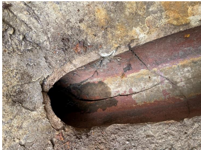
Photo 10: Cracking to the pipework to the drainage run which passed below the Kitchen extension. Within the inspection chamber adjacent to the back door
