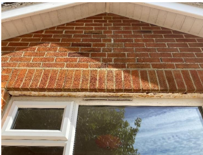
Photo 9: Corroded metal lintel above the Front Bedroom window
