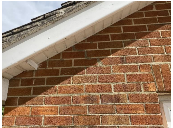
Photo 8: Repointing to the wall above the West side of the Front Bedroom window
