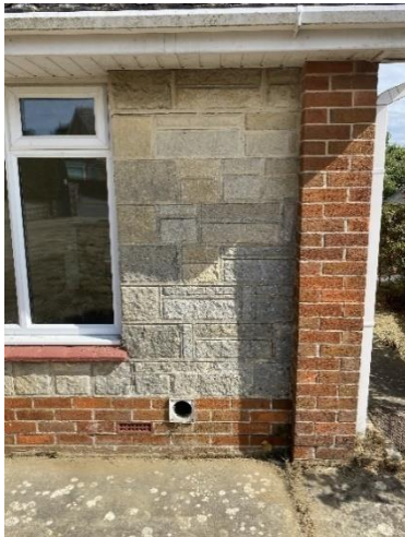
Photo 5: Cracking to the stonework to the front elevation of the Reception Room
