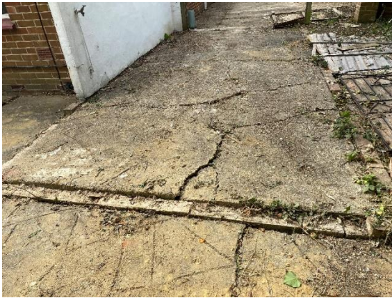
Photo 7: Crack to the concrete slab adjacent to the West side elevation of the property – 13th July 2022
