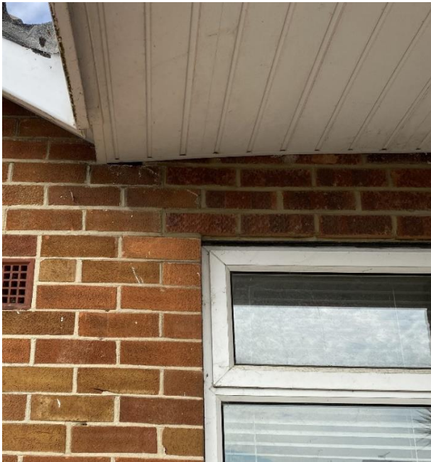
Photo 3: Wall above the window to the East side elevation of the Kitchen extension. At the junction between the main property and the extension to the rear - 13th July 2022
