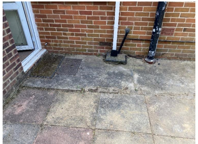
Photo 36: Foul and surface water downpipes with gulley and inspection chamber against the rear elevation of the main property, to the West side elevation of the extension
