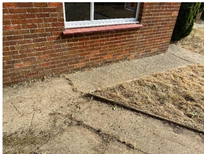
Photo 22: Damp proof course only 10mm above the path which falls towards the front of the property. Surface water was thought to pool on the path against the building
