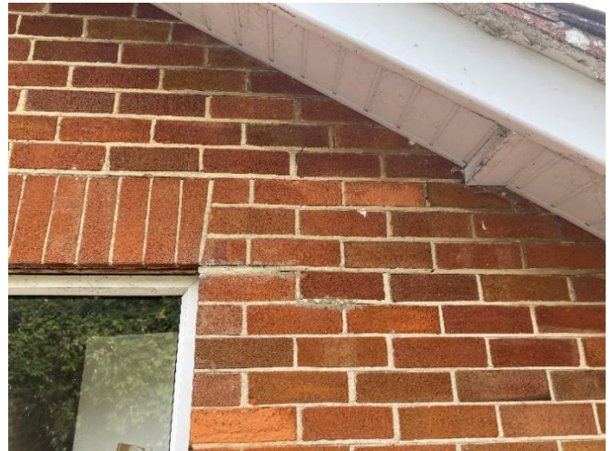
Photo 12: Cracking and repointing above the South side of the Middle Bedroom window
