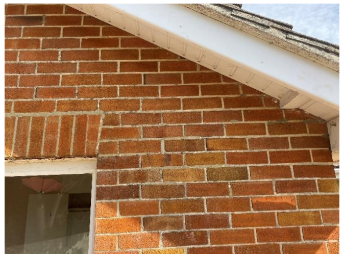
Photo 10: Repointing to the wall above the East side of the Front Bedroom window
