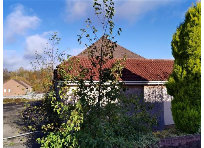
Figure 6 – View of southwestern corner of the building, looking north towards hardstanding area at the back of the building.
