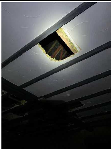
Figure 15 - Hole in the roof at the north of the building.
