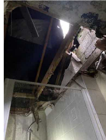
Figure 12 - Hole in roof within bathroom located at the south of the building.
