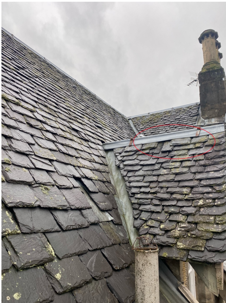
5. Rear. West facing elevation. Illustrative of roof-state.
