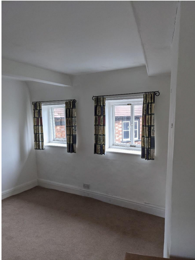
Figure 28: First floor bedroom, largely featureless, with two casement windows looking out from the south eastern elevation. Two covered timber beams can be seen on the ceiling.
