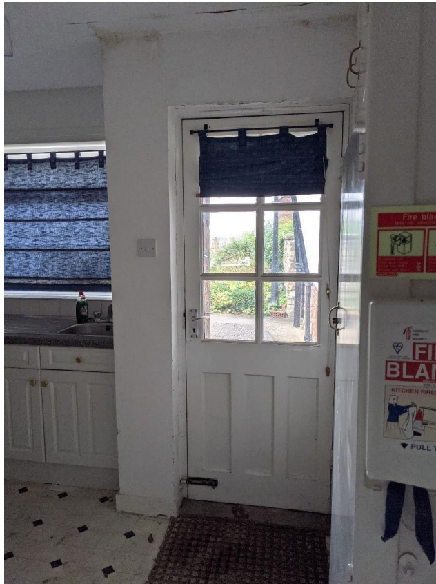
Figure 20: A half glass, three vertical panelled door set into the southern elevation of the rear extension. To the right of the door are a set of fitted cabinets that may be contemporaneous with the original fabric of the extension.
