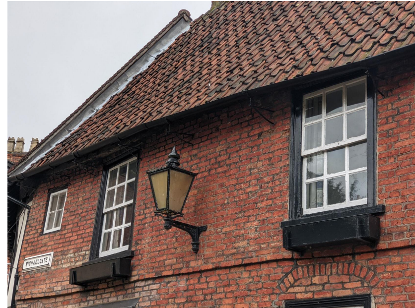
Figure 17: Cast Iron lamp reminiscent of the Victorian style added to the northern elevation in the late 20th century. The window boxes below the first floor 18th century sash windows are also late 20th century additions. The two brick width string course can be seen just below the window boxes. 42 Michaelgate is roofed with clay pantiles.
