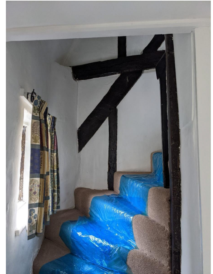
Figure 30: Timber frame construction, including a brace, tie beam and studs, of the party wall between 42 Michaelgate and the Harlequin in the first floor to second floor stairwell.
