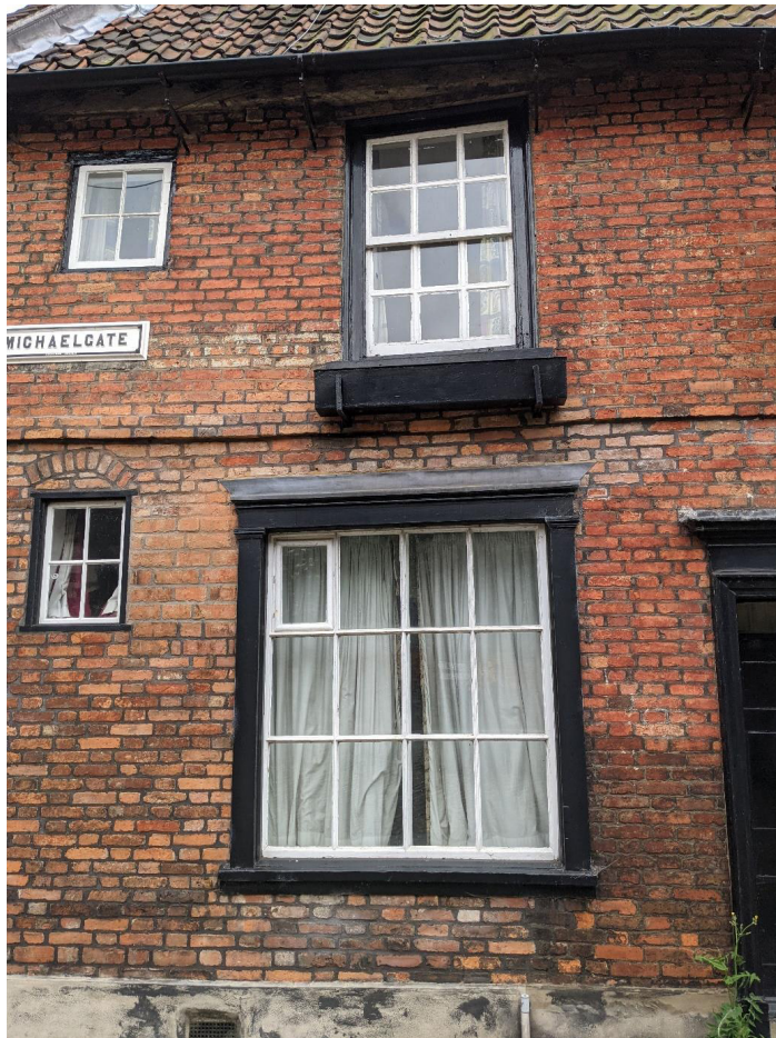
Figure 18: Close up of the 18th century glazed barred shop window, framed by two pilasters topped with decorative comices. The 2018 area of repair can be clearly seen below the first floor casement window.
