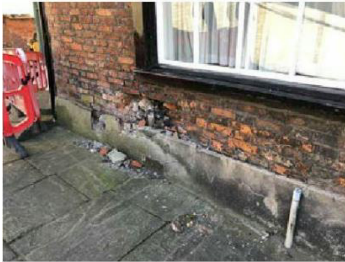
Figure 14: Damage to the base of the north elevation, below the 18th century shop window, caused by a vehicle impact in 2018.
