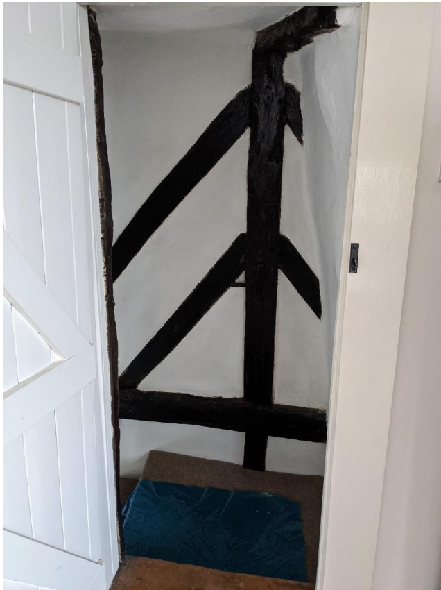
Figure 31: Further example of timber frame of the Harlequin party wall, showing two sets of angled braces attached to a central king post.
