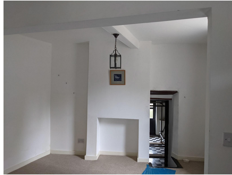
Figure 23: The south west half of the ground floor, the central 18th century fireplace was blocked in the 20th century. To the right of the chimney breast is a small flight of stairs leading into 40 Michaelgate. Above the fireplace is a covered timber beam.
