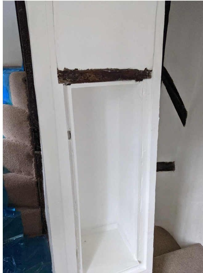
Figure 26: A possibly 18th century fitted cabinet, with door removed, into the first floor landing wall between ground to first floor and first floor to second floor staircases.
