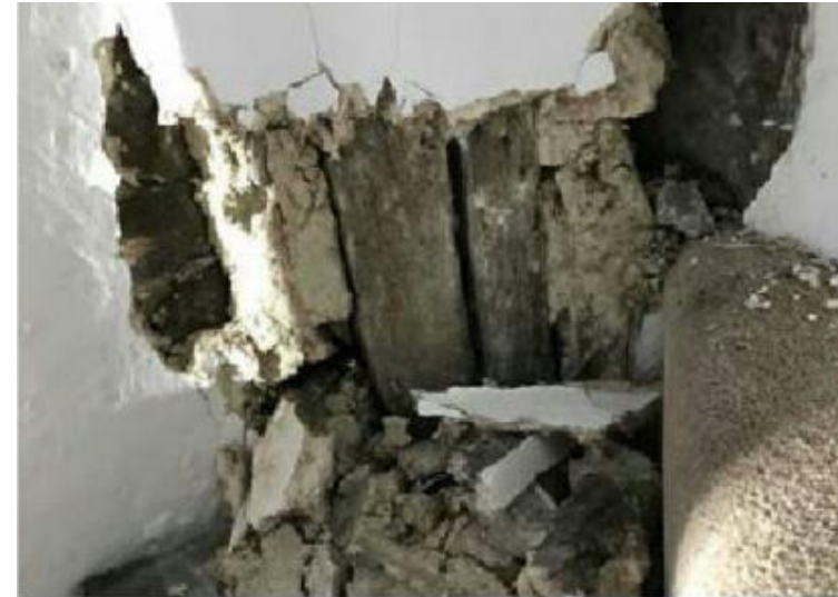
Figure 15: Internal damage to the ground floor to first-floor staircase caused by a vehicle impact in 2018. The impact has punctured the wall causing the lime plaster to come away from the wooden timber frame of the party wall between the Harlequin and 42 Michaelgate.
