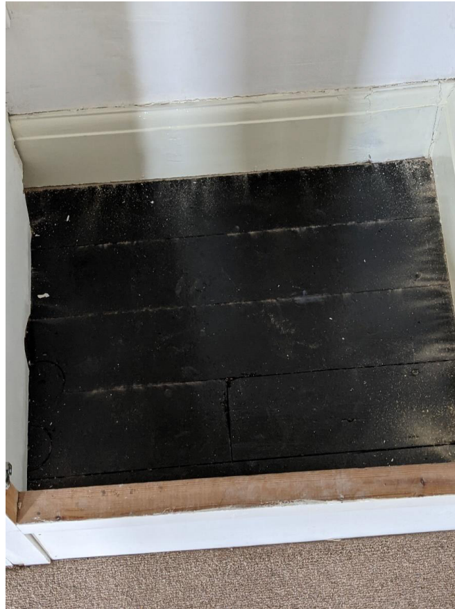
Figure 29: Example of 19th century stained floor boards found throughout the first floor below the carpet.
