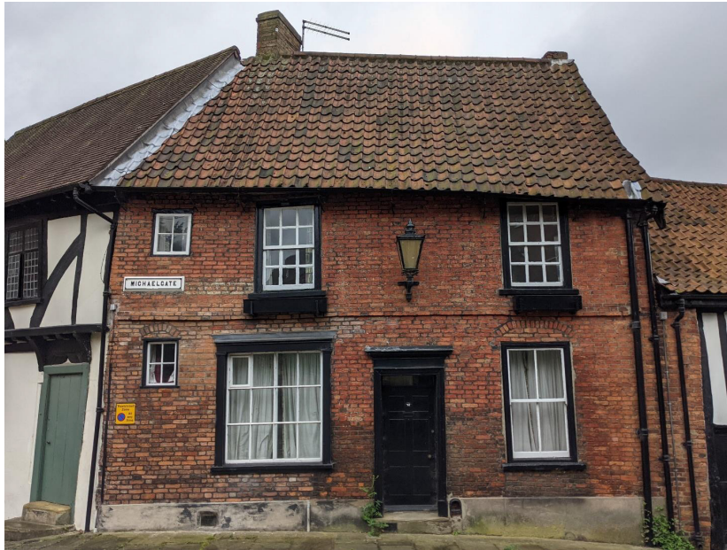
Figure 16: Northern elevation, street facing, of 42 Michaelgate constructed in red brick laid in Flemish bond atop a stone plinth with a brick string course dividing the ground and first floor. The 2018 area of repair can be seen on the left hand section of the ground floor elevation, extending from the Harlequin party wall to the door. The chimney stack has been largely removed on the western gable and the chimney pot has been removed at some from the eastern gable stack. There are two small 18th century casement windows with relieving arches inserted into the ground and first floor wall of the staircase. Left of the door is a 18th century glazing bar shop window adorned with pilasters and cornices, while on the right of the door is a plain sash window again with a relieving arch. On the first floor are two 18th century sash windows. Above the door is a late 20th century cast iron lamp with cast iron bracket. The central beaded panelled door is topped with a small hood and transom overlight.
