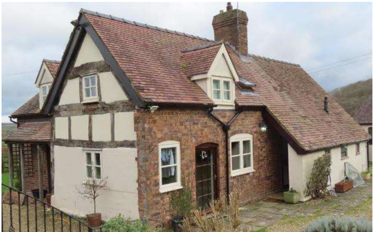
Photograph 4. Exterior. Left: parts of the Northwest elevation of Section A. Centre and right: Southwest elevation of Section A. Right: Southwest elevation of Section B.
