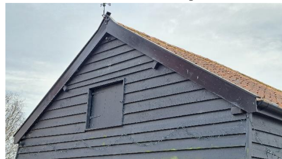
Photo 2 View of north west corner showing good condition weather board and barge boards.
