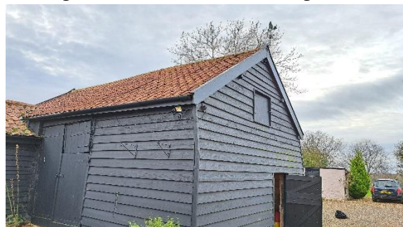
Photo 1 View of East and North Elevations of Barn showing double barn door and north gable wall.
