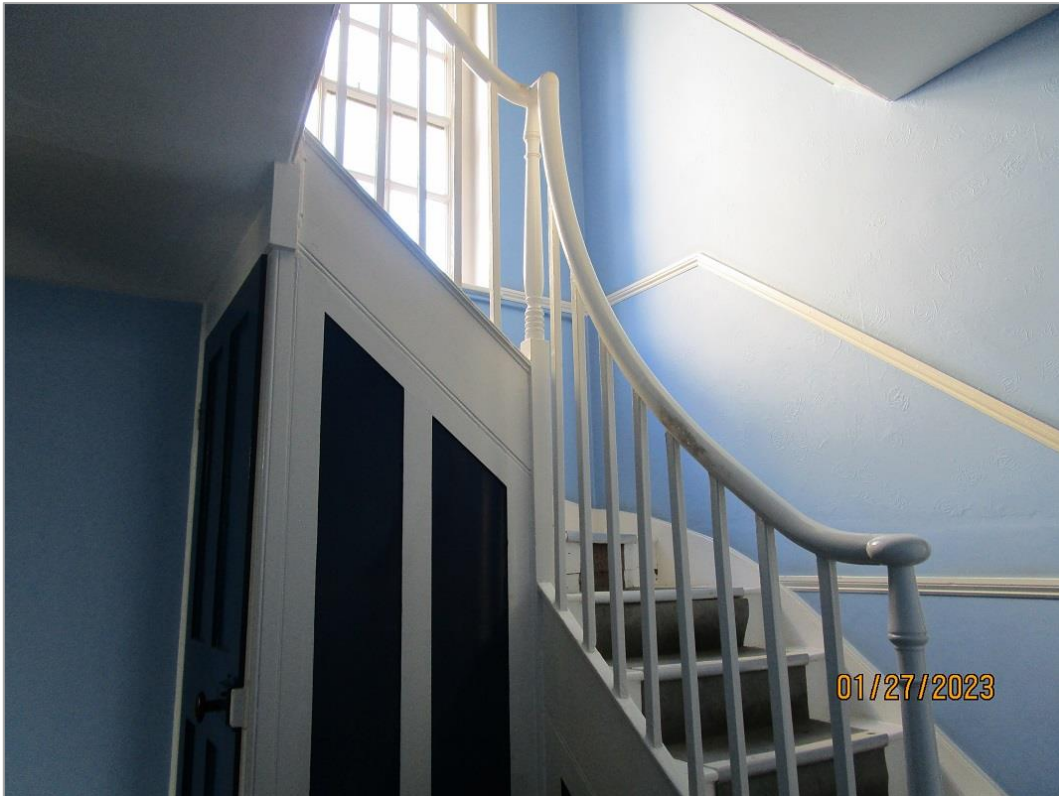
Fig. 35: The stair to first floor is of late C18/early C19 character, with closed string, stick balusters, turned newels and swept handrail, all painted. The dado rail on the wall is probably modern. The stair is lit by a large multi-pane sash window. Below the stair is a winding stair to the cellar.
