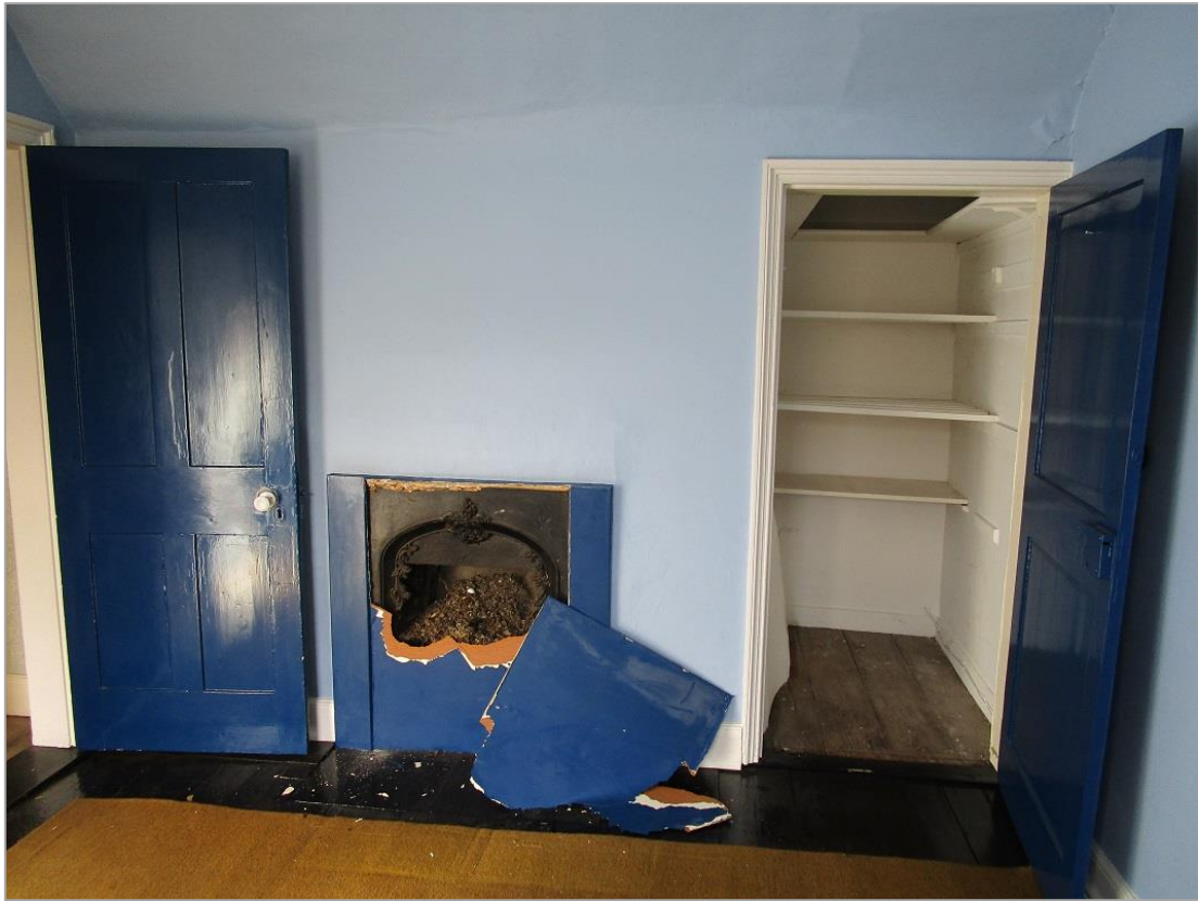
Fig. 28: Four-panelled door, elaborate cast iron C19 fireplace (minus top of surround) and cupboard with two-panel door, first floor front bedroom.
