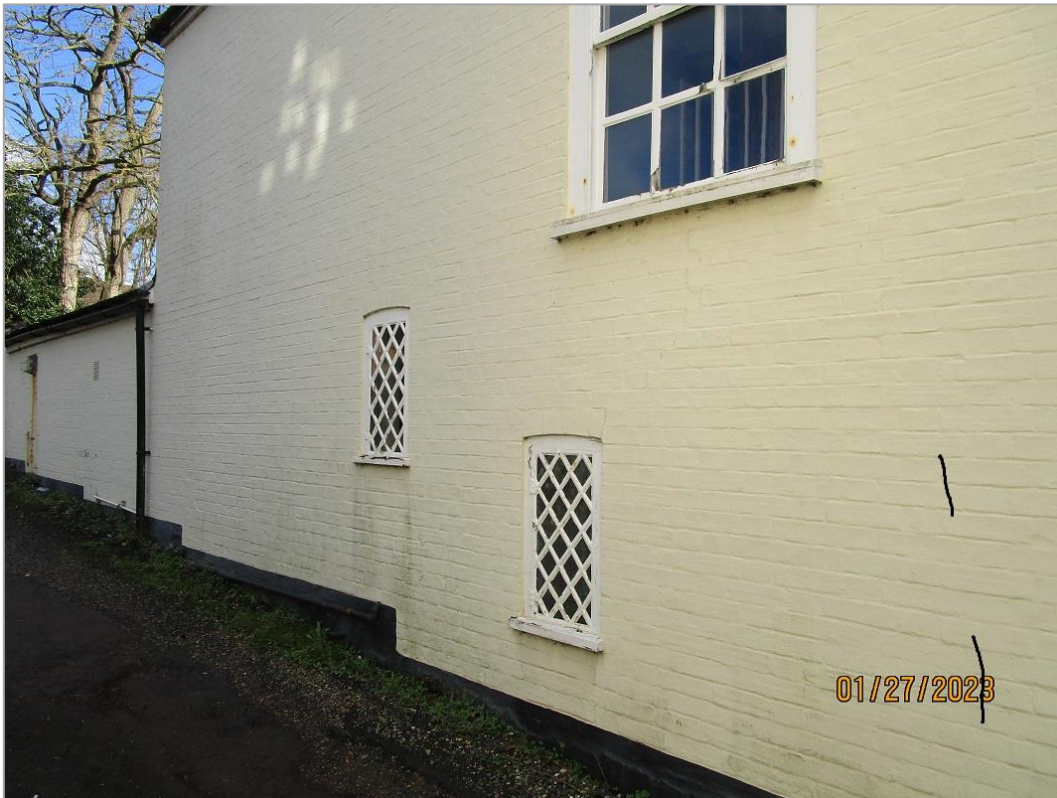
Fig. 11: Facing the side access is a C18 two-storey rear range to no. 14, of painted brick and with a large flush framed 6-over-6 glazing bar sash window lighting the staircase. Below are two metal casement windows with diamond lattice panes, the nearer (lower) one lighting a stair to the small cellar, the further one a ground floor WC.
