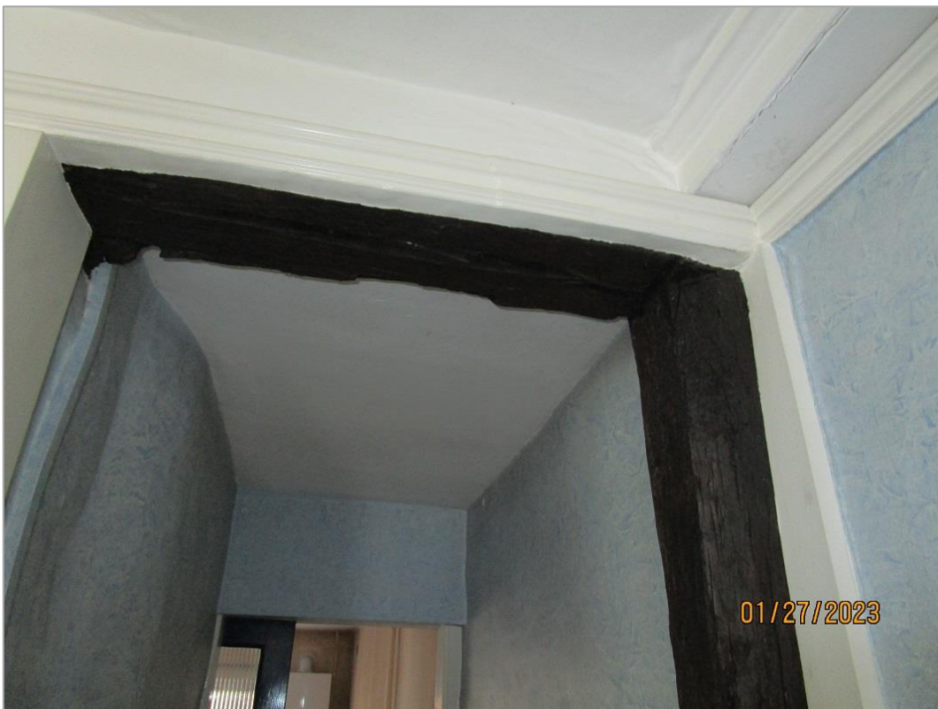
Fig. 21: Exposed timber framing alongside the chimney breast in the northeast corner of the room to right of entrance hall.
