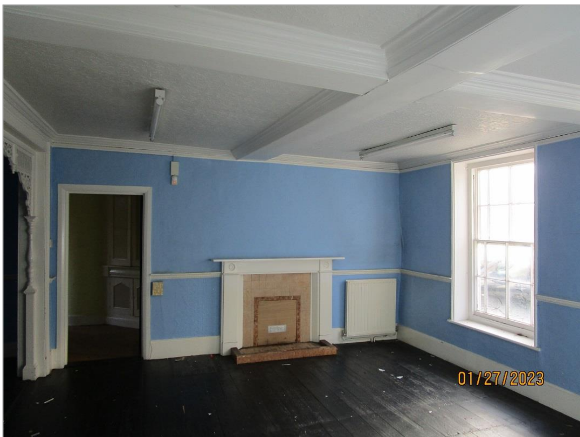
Fig. 32: The large room to the right of the hallway has boxed-in beams with C19 mouldings to the boxing, timber fireplace with roundels and C20 tiled inset, boarded floor, dado rail (probably C20) and embossed paper lining the ceiling. Decorative surround to alcove to left, shown in more detail at fig. 33.
