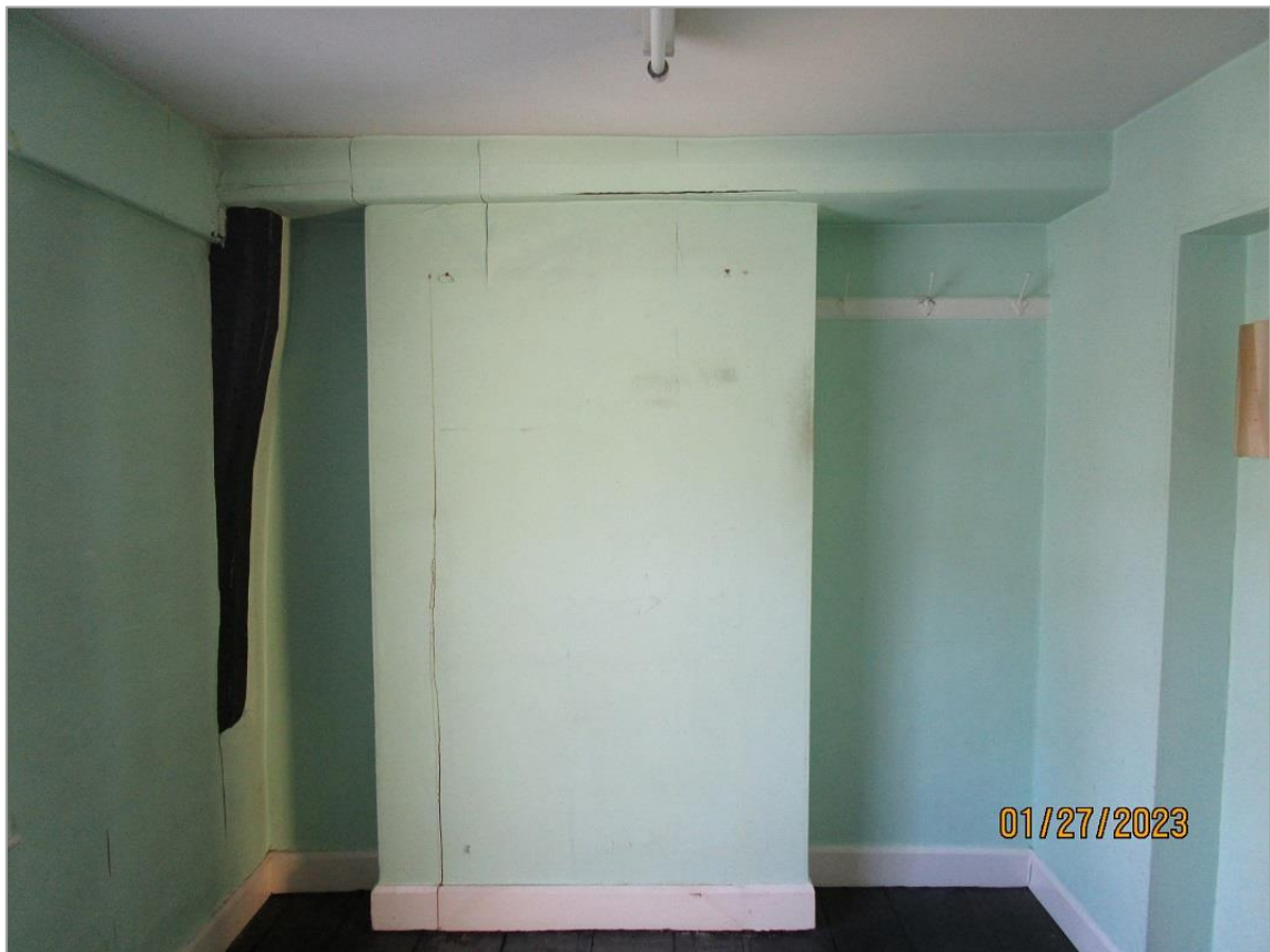
Fig. 40: Chimney breast, jowled post and boxed-in beam, first floor rear room, front range
