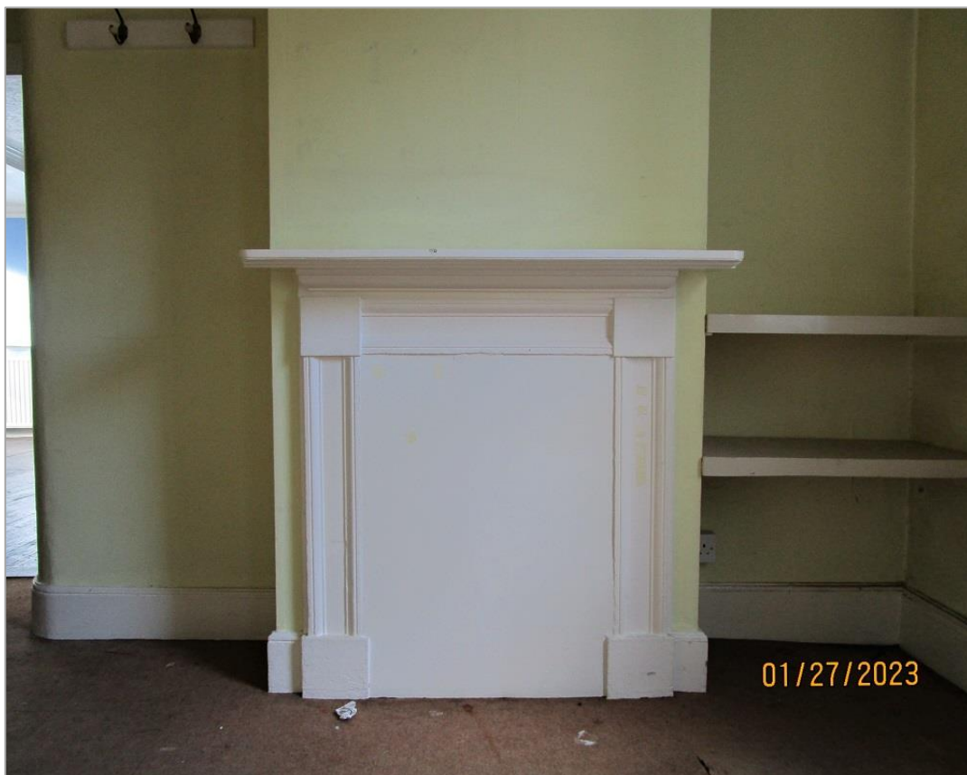
Fig. 23: Boarded-up C19 timber fireplace in rear ground floor room of front range
