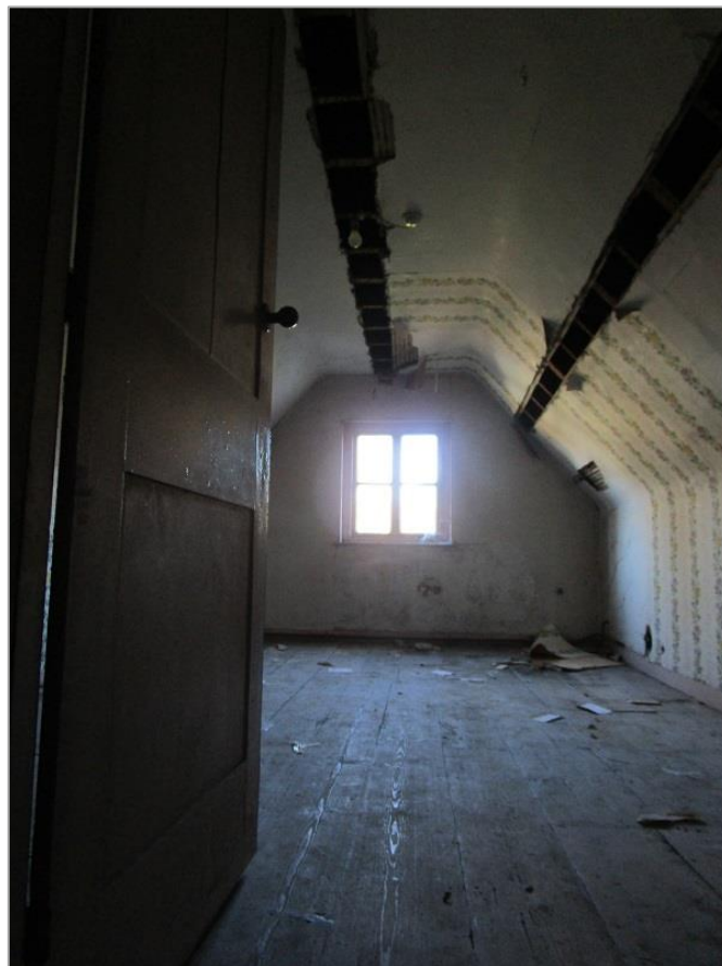
Fig. 29: A second floor room is reached via a steep stair with two-panel door at the top.
