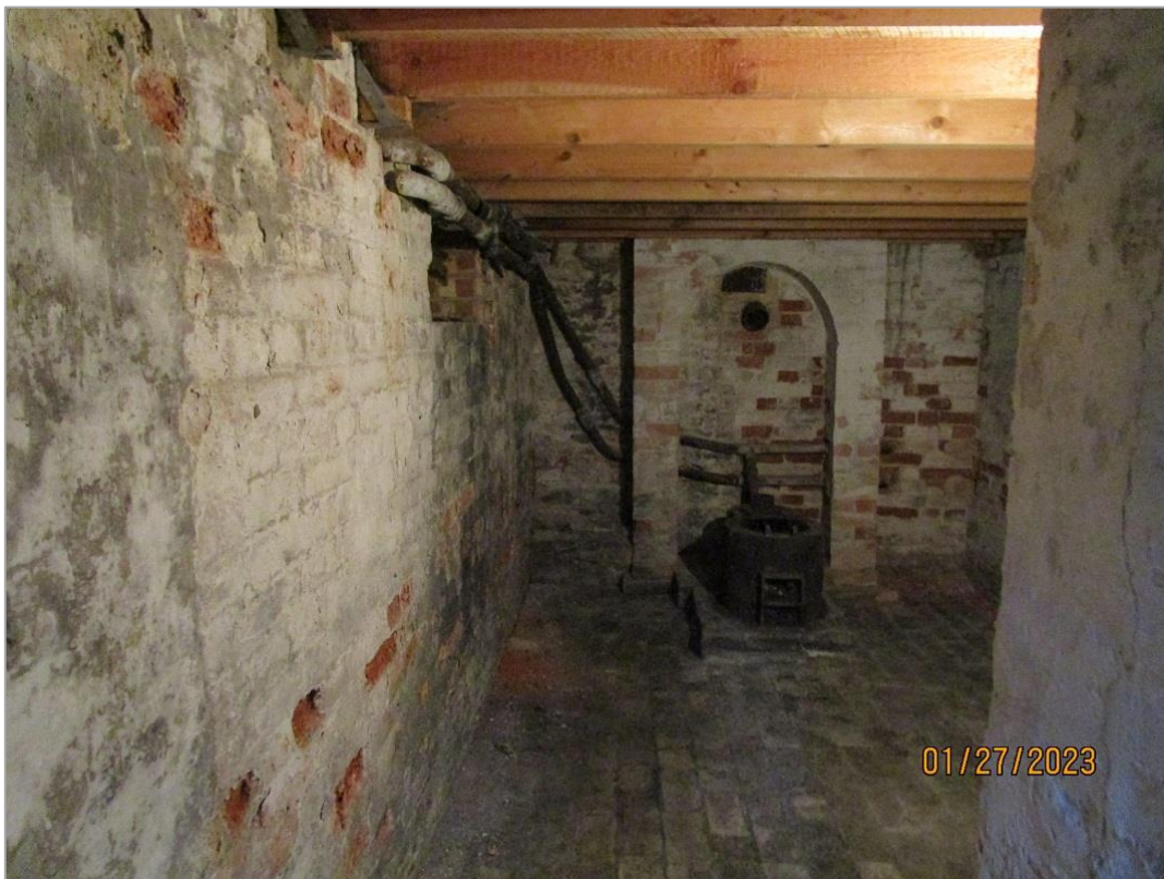
Fig. 34: The cellar is reached by a winding stair under the main stair and has a brick floor, whitewashed brick walls and the remains of a cast iron heating apparatus in front of the stack. Recesses for wine racks or storage on south side. The floor joists above have been renewed in the C20.
