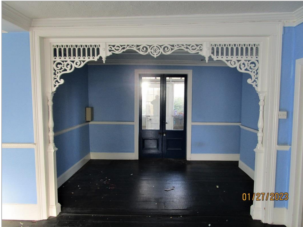
Fig. 33: Decorative timber surround (late C19) to opening to rear room on ground floor. Beyond, French doors now lead to C20 conservatory. Below this rear room is a cellar (fig. 34)
