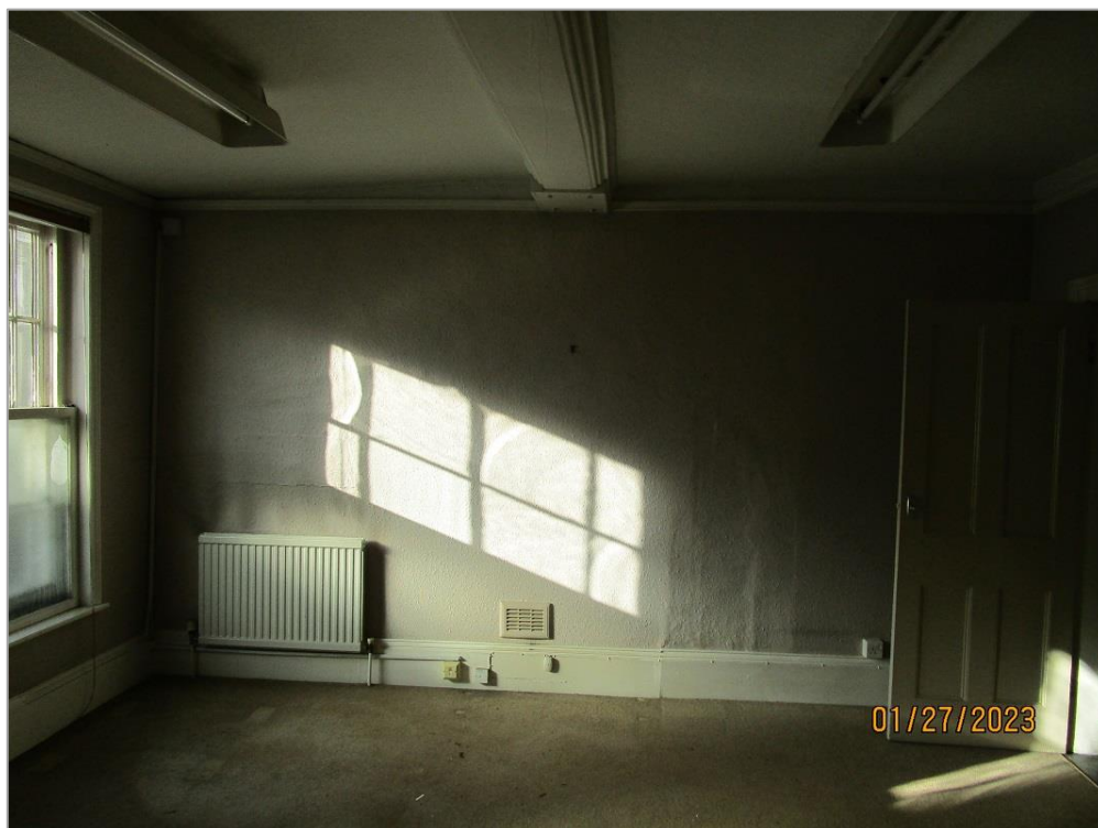
Fig. 17: The room to the left of the entrance hall has a simple cornice and moulded skirting of C19 character. The fireplace opening has been blocked. Above is a C17 roll moulded and chamfered oak beam, painted white (see also fig. 18)
