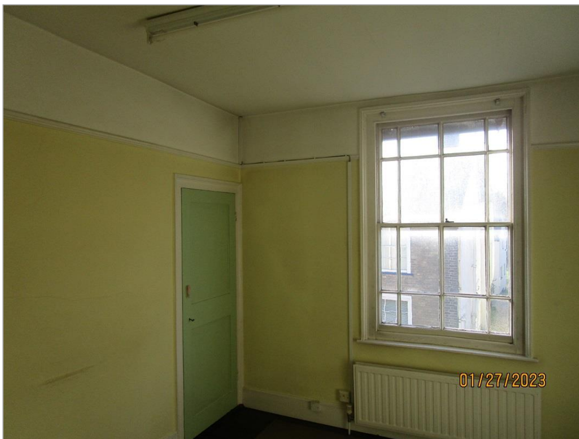
Fig. 42: Front bedroom with two-panel door to cupboard to right of chimney breast
