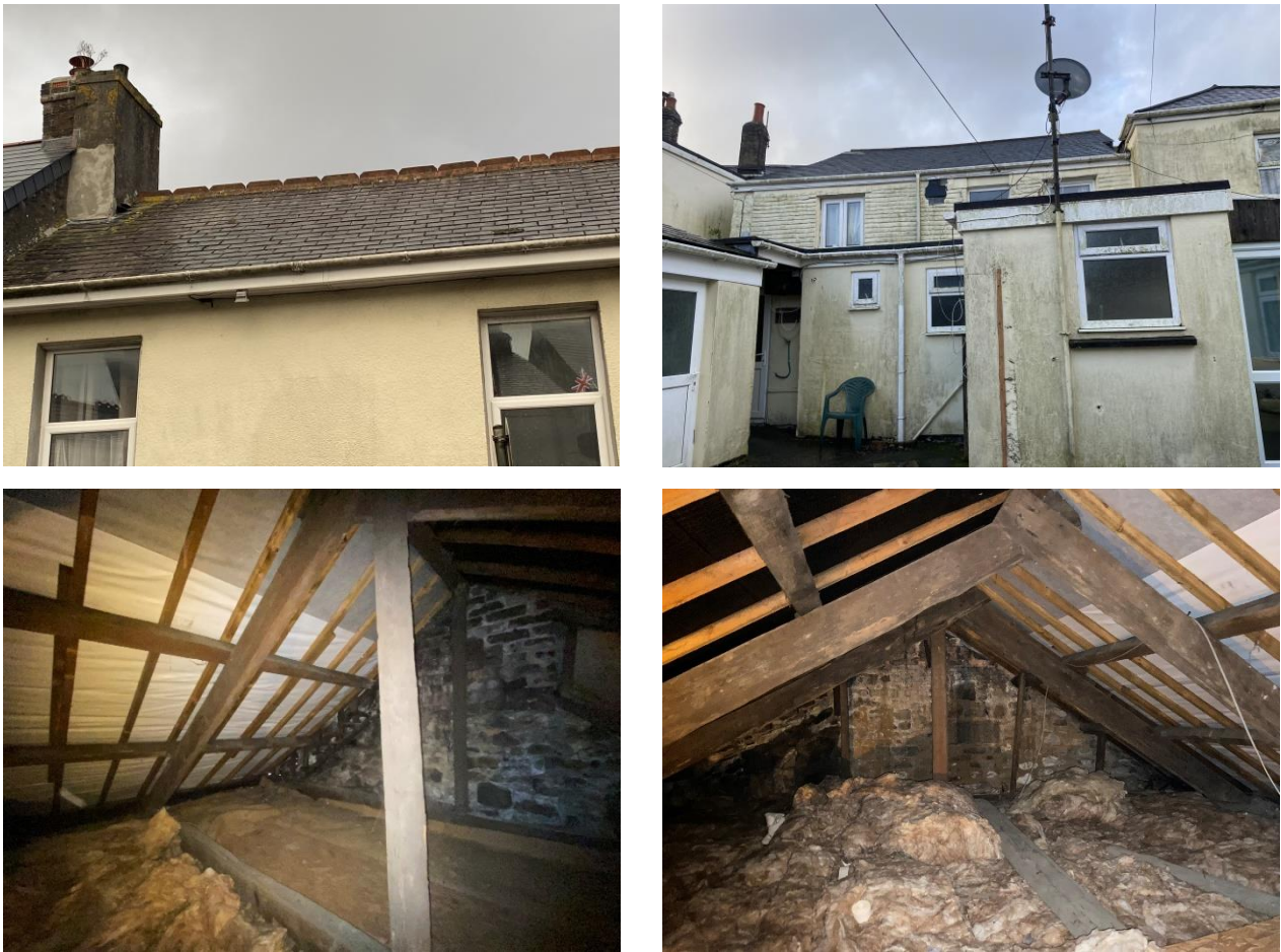
Figure 2: The roof on the front of the pub (top left), the rear aspect (top right) and the internals of the roof void to the west (bottom left) and east (bottom right).
