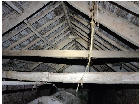
Photo 14. An internal view of the western section of the Single Storey Barns (photo taken at night).
