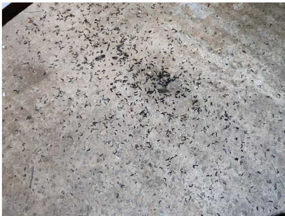
Photo 21. The cluster of lesser horseshoe bat droppings and insect feeding remains within the ground floor southern room.
