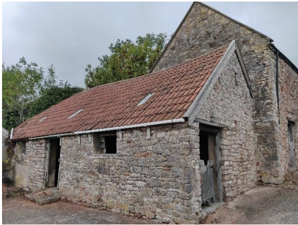
Photo 11. The southern and eastern elevations of the Single Storey Barns (eastern section).
