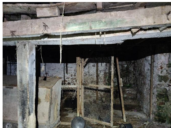
Photo 10. An internal view of the Main Barn showing the floor and northern platform area.
