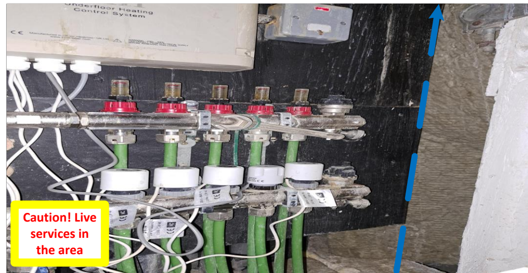
11 First Floor Bedroom Riser
