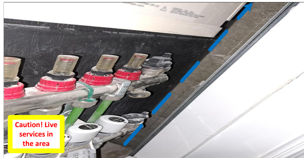
9 Ground Floor Lounge Riser
