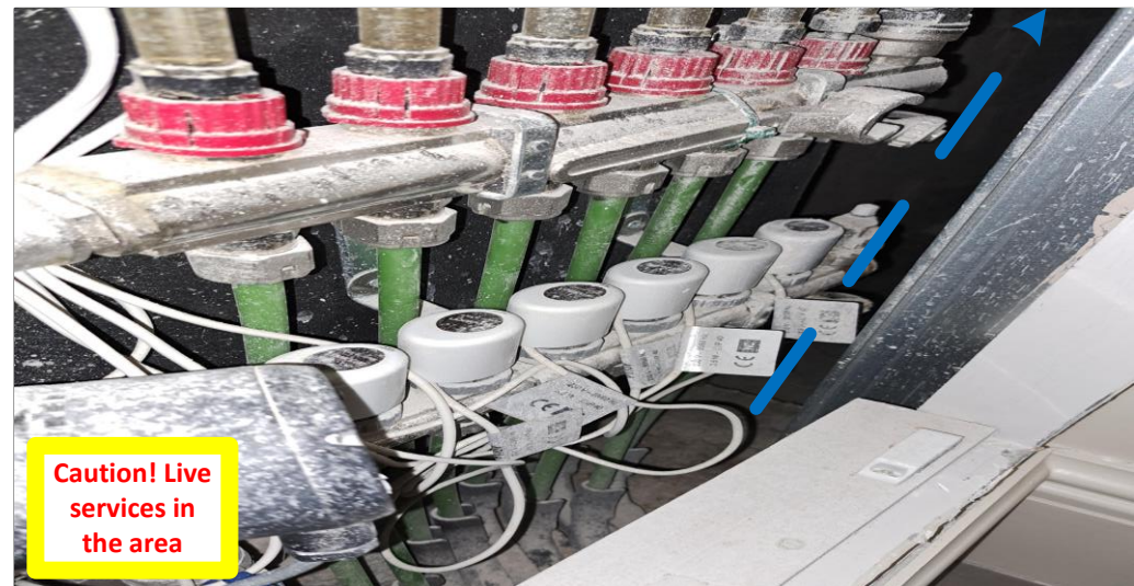
7 Ground Floor Lounge Riser
