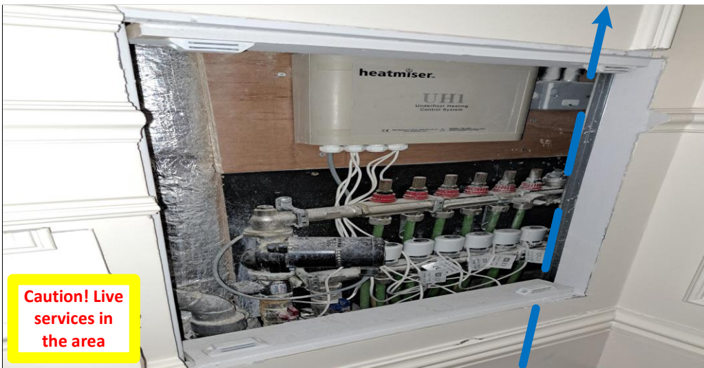
6 Ground Floor Lounge Riser
