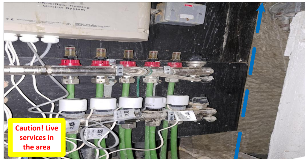
13 Second Floor Bedroom Riser
