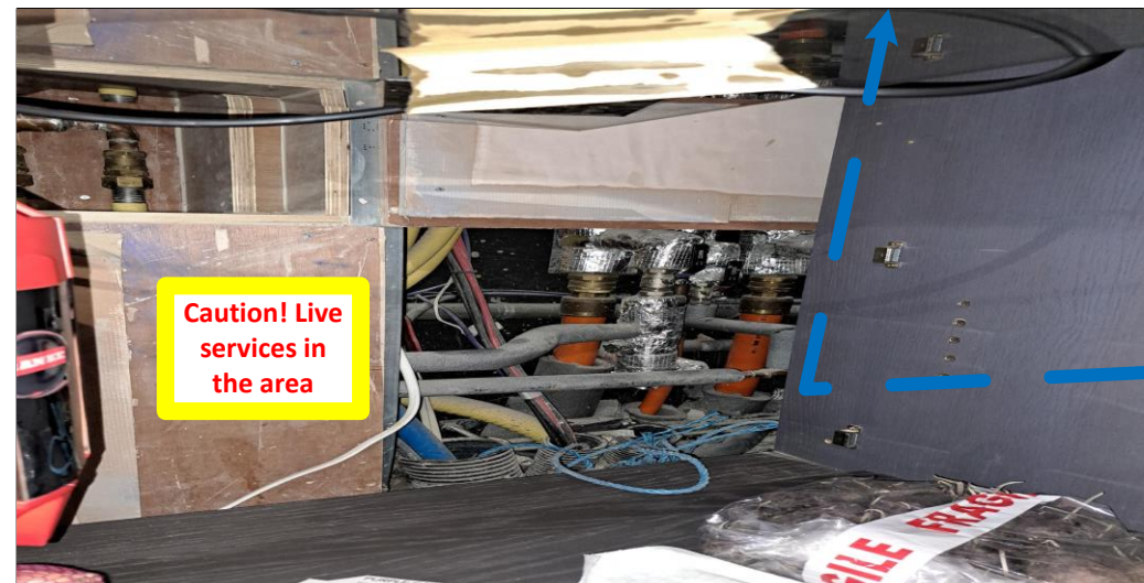
12 Kitchen – the 2f cable will then go up through to the next floor from behind
