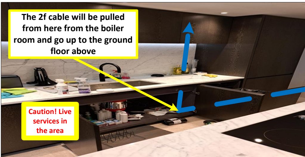
11 Basement Kitchen – the 2f cable will be pulled through from the boiler room from here
