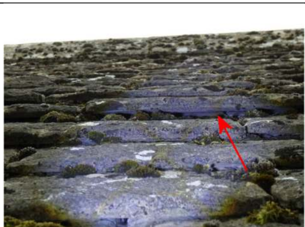
Photograph 6. Example of an opening under the slates on the west-facing roof pitch
