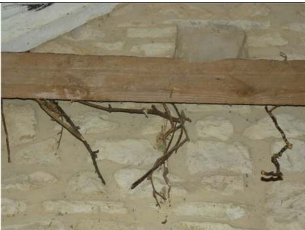
Photograph 17. Possible nesting material in the room at the southern end of the building
