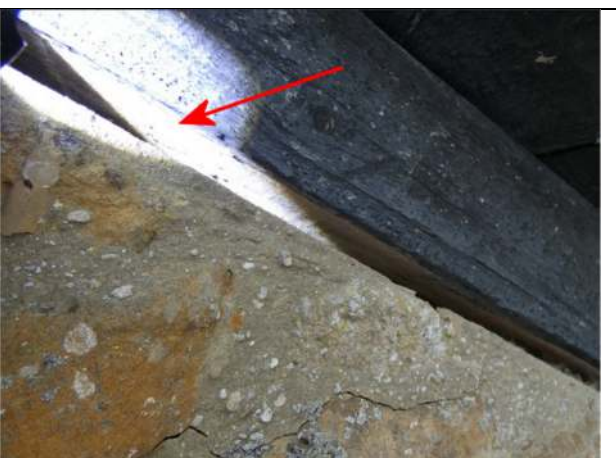
Photograph 10. Crevice between the gable rafter and the north gable wall
