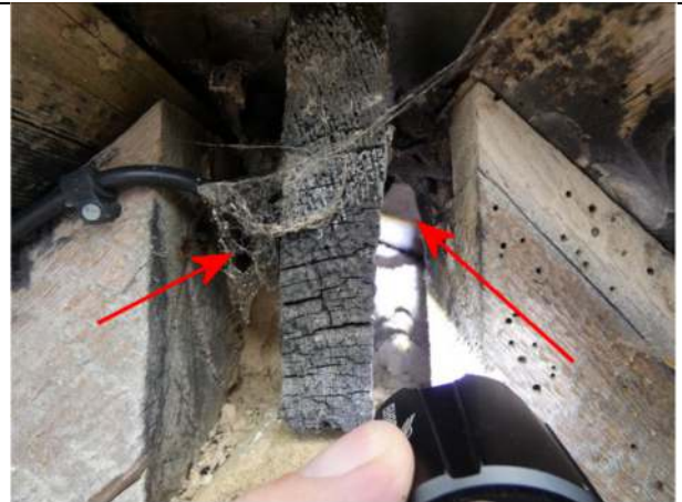
Photograph 8. Crevices on either side of the protruding ridge board at the apex of the south gable wall
