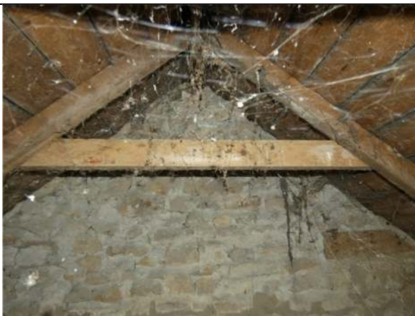
Photograph 15. Example of dense cobwebs under the ridge in the central and north bays
