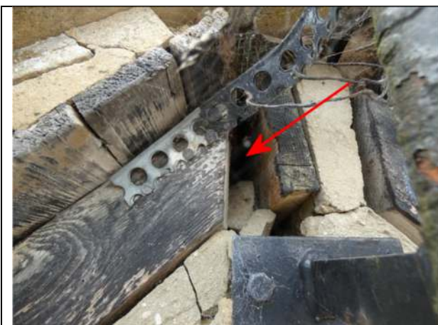
Photograph 9. Crevice to the side of the protruding ridge board at the apex of the north gable wall
