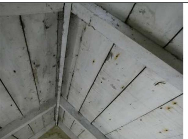
Photograph 12. The painted timber sarking in the room at the southern end of the building
