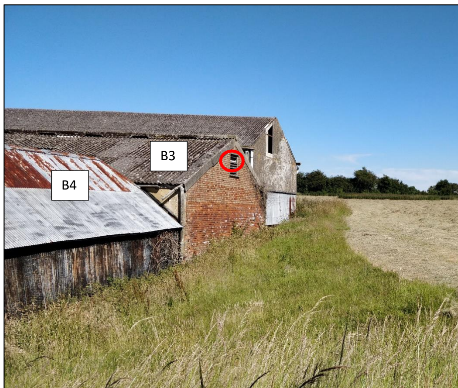
Photo 8.1: Proposed location of little owl box and perch (red oval) on southern gable end of Building B3, once existing ventilation has been filled in as part of conversion works.
