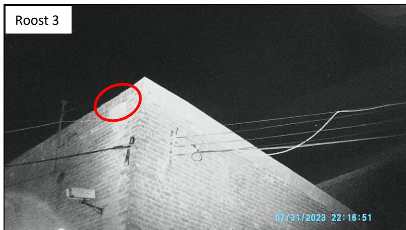
Photo A5.3: Location of emergence point from beneath corrugated metal roof edge on 10.07.2023 for Roost 3, common pipistrelle day roost (Building B2, view from IR Whisker camera). Note the date stamp is incorrect and should say 17 th July 2023.
