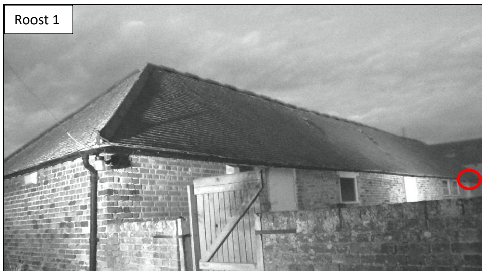
Photo A5.1: Location of emergence point under bottom row of tiles or from eaves on 03.08.2023 for Roost 1, common pipistrelle day roost (view from IR Canon camera).
