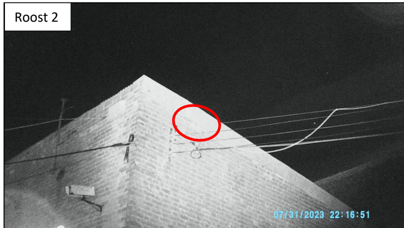
Photo A5.2: Location of emergence point from under lead flashing on 10.07.2023 and 17.08.2023 for Roost 2, common pipistrelle day roost (Building B2, view from IR Whisker camera). Note the date stamp is incorrect and should say 17 th July 2023.
