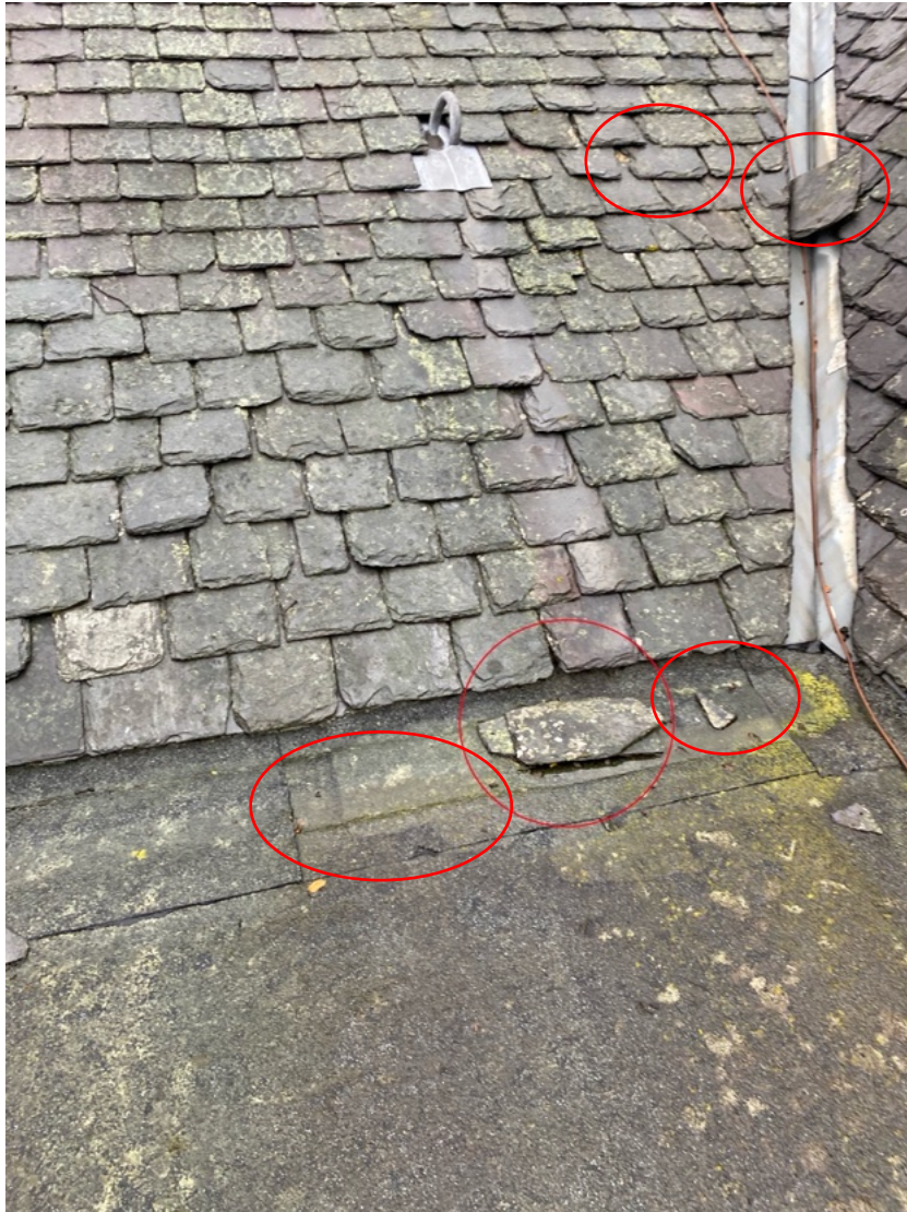
8. Roof valley. Damage at former repair site.
