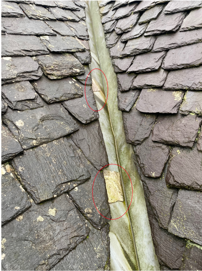
6. Rear. West facing elevation. Damaged lead work
