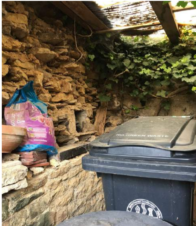
Internal view of right hand space prior to collapse
