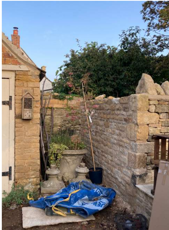
Right hand side of outbuilding (collapsed structure has been cleared away)
