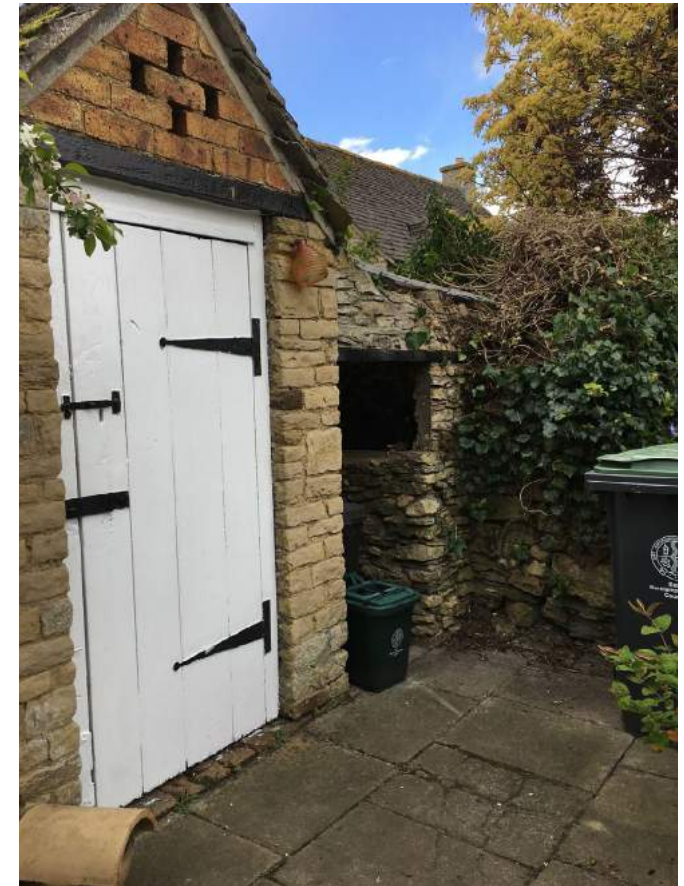
External view of right hand space prior to collapse
