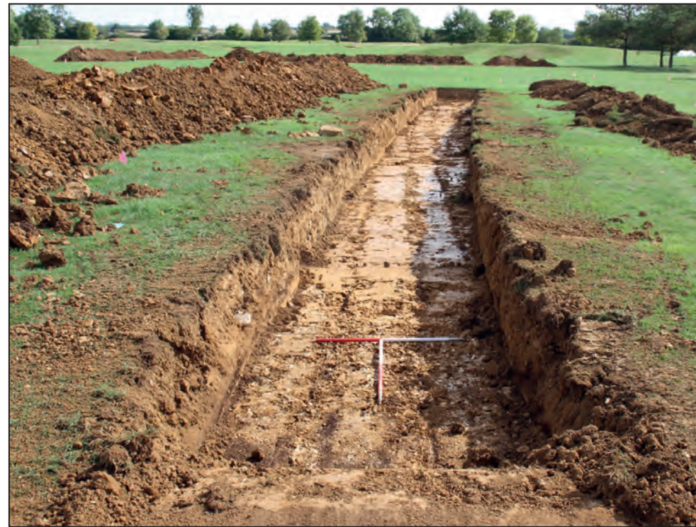
Trench 6, looking east, showing depth of made ground and previous drainage impacts (1m scales)
