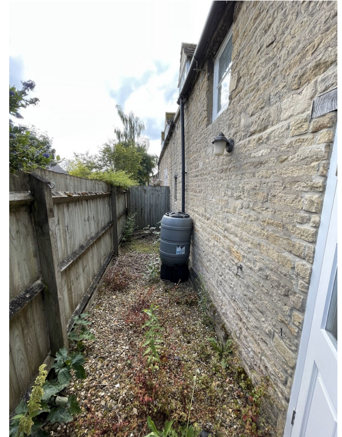
View of the rear courtyard showing drainage into water butts—no connection into appropriate soakaway
