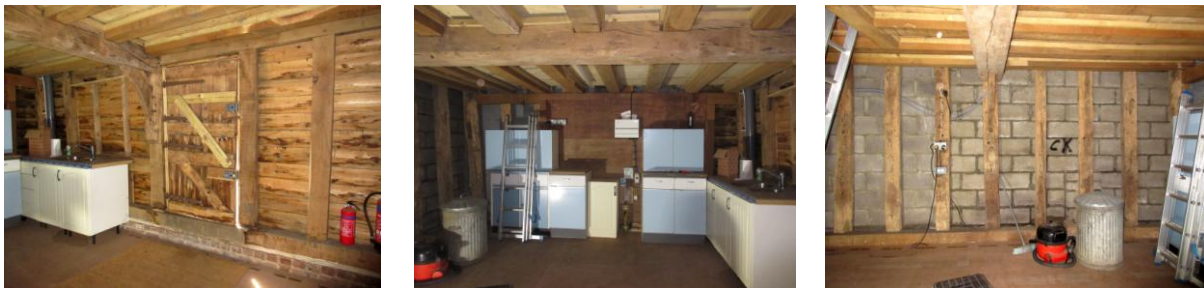
SE bay: Left: looking S showing stable door with concrete cill on re-built brick plinth beneath replacement sole plate and replacement studs to SE of door; Centre: looking SE showing original binder (chamfered) and replacement upper floor joists, SE end wall lined with ply; Right: looking NE showing original studs set in replacement sole plate
