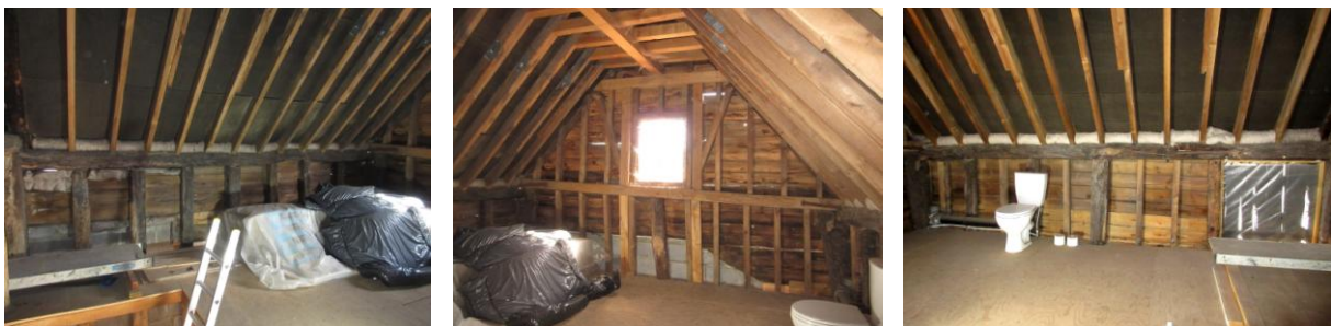
SE bay: Left: looking E showing upper part of SE wall with smoke blackened studs and wall plate and replacement rafters in NE roof slope; Centre: looking SE showing replacement framing in SE gable wall apart from central stud and inserted window; Right: looking SW showing replacement rafters in SW and 3 original remaining studs, original wall plate, loading door (SE of pair) on right, replacement loft floor with stair well (no staircase) supported on replacement joists
