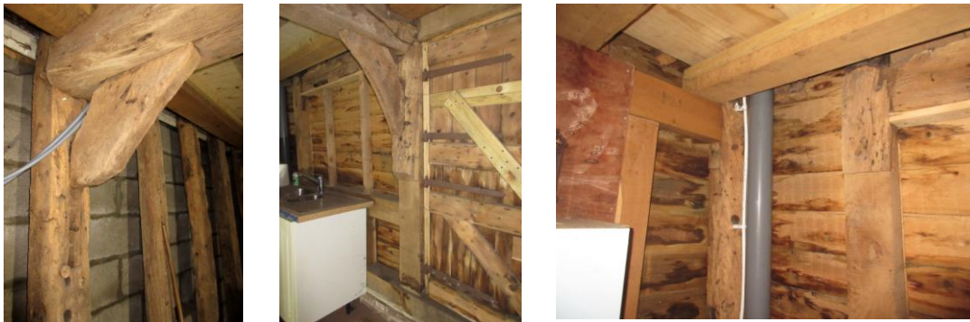
SE bay; Left: reduced brace at NE end of binder; Centre: complete brace at SW end of binder bolted onto replacement post; Right: SW corner showing original corner post with replacement framing on rear SE wall to left and replacement floor above
