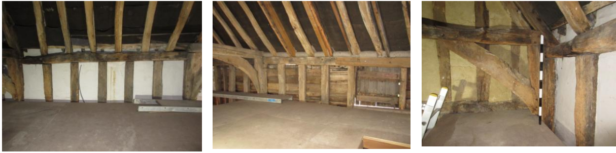
NW bay; Left: NE wall with original rafters, wall plate and studs; Centre: SW wall looking S showing replacement rafters and new section of wall plate above loading door; Right: N corner showing jowelled corner post, tiebeam and arch brace in front of rear wall of 2 Bridge Street
