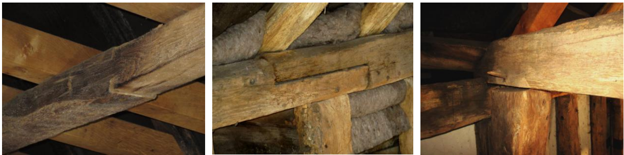
Left: bridled, edge halved scarf in collar purlin in middle bay; Centre: edge halved scarf in NE wall plate of middle bay; Right: detail of NW side of junction between NW and middle bays showing jowelled main post supporting wall plate and NE end of tiebeam which has a plain chamfer with flat stop
