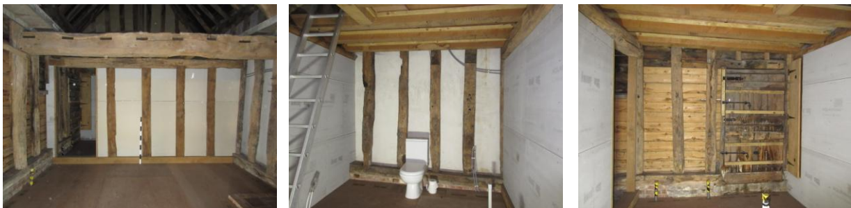
Left: looking NW from middle bay showing dividing wall original studs set in replacement sole plate, doorway leads into NW bay; Centre: NW bay looking NE showing replacement upper floor and plaster board lined walls; Right: looking SW showing stable door, original studs and replacement weather boards
