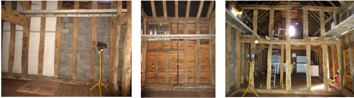
Middle bay; Left: looking NE showing original studs and sole plate with concrete block wall behind, brick standing in front; Centre: looking SW showing replacement studs beneath loading door; Right: looking SE from middle bay showing partition wall with infill removed
