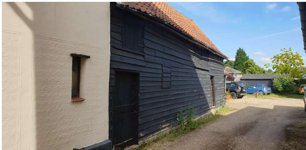
Barn viewed from within the site access, looking east along the flank wall of No. 2
