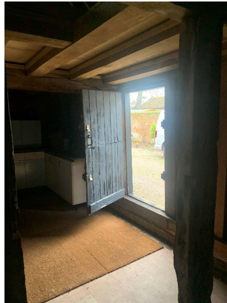
Photograph of the entry and example of some of the works that had been undertaken (new floor and beams on 1 st floor)
