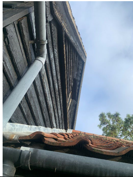
Photograph of edge tile with missing concrete allowing potential points of ingress. On the adjoining single-story Barn.
