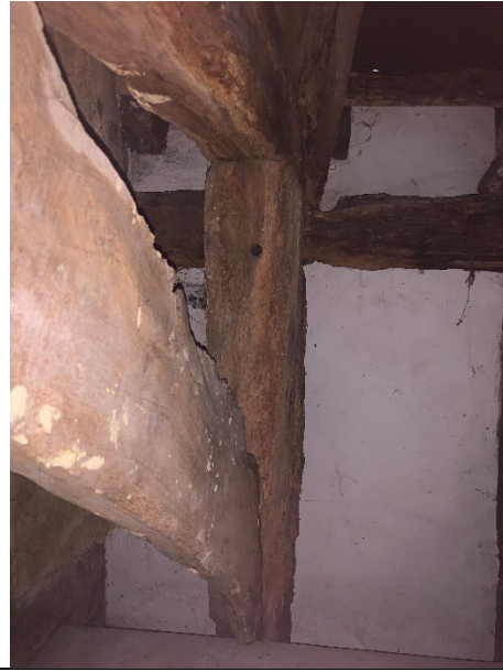
Photograph of exposed rough beams with gaps around the joins.
