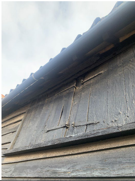
Photograph of single skin timber cladding walls on the front of the building and doors on the first floor with some potential points of ingress under the cladding and around the door.
