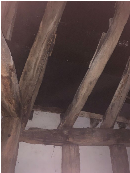
Photograph of exposed rough beams with gaps around the joins and lifting roofing membrane.
