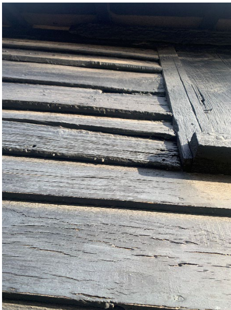
Photograph of single skin timber cladding walls on the front of the building with some potential points of ingress under the cladding.
