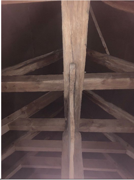
Photograph of exposed rough beams with gaps and splits on the beams of pitched roof with the nonbreathable membrane.
