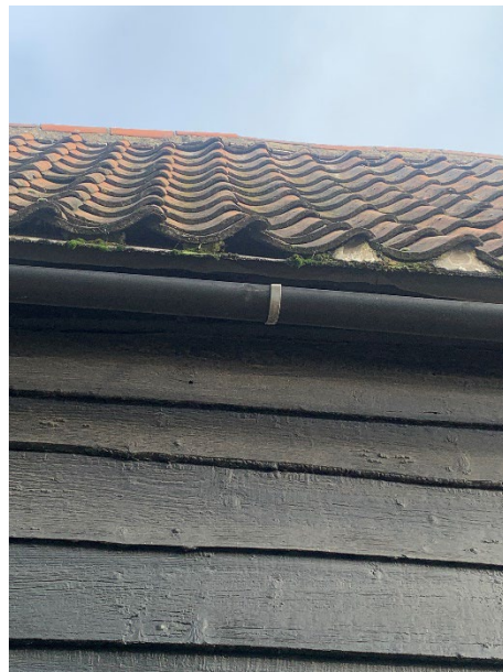
Photograph of edge tile with missing concrete allowing potential points of ingress.
