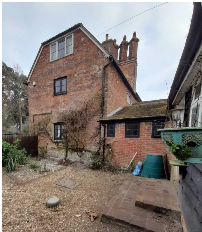
Fig. 11: View, looking east, of the right-hand element of the north-west elevation, and single-storey extension to the right.
