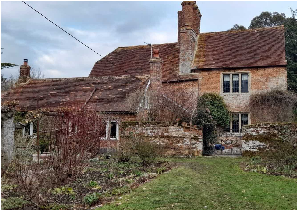
Fig. 8: The south-west elevation of Tadley Place Farmhouse, with the nineteenth-century single-storey extension in the foreground.
