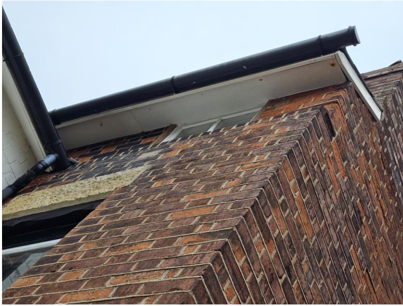
Photograph 3: Close up of the sealed soffit to wall top join where the north elevation dormer will be located
