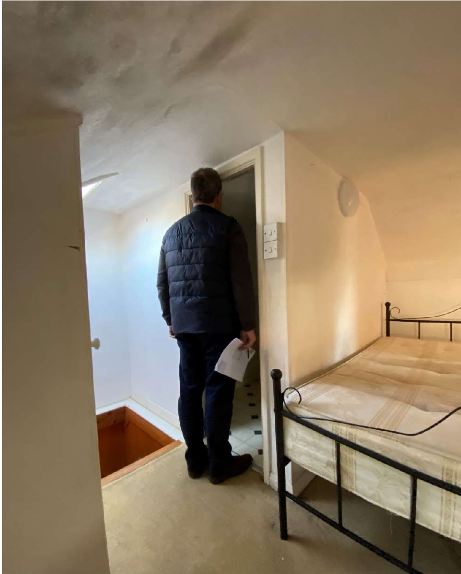
Photograph 11: Similar to photograph 10, indicating the low ceiling height and limited headroom at second floor level
