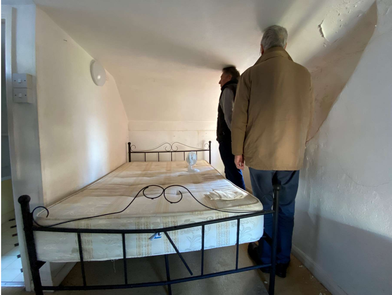
Photograph 10: Existing bedroom at second floor level. The existing ceiling height is lower than that in a typical dwelling, leaving very little head room. The ceiling height reduces further towards the head of the bed, following the roof slope
