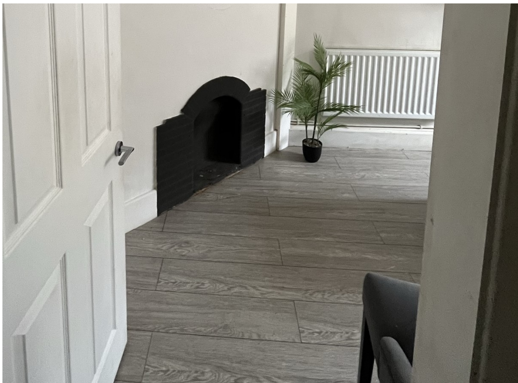
6. The modern corner fireplace in the first floor front room, which it is proposed to cover over, may represent infilling of an earlier, larger opening.
