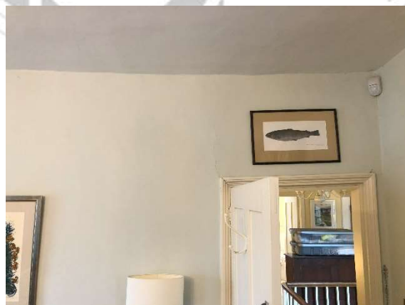
Slight cracking to corner of door at opposite end of room
