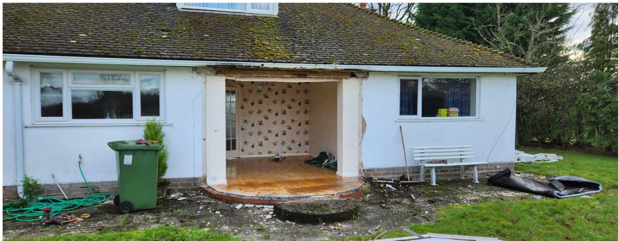
Fig.4 – Recent photograph of rear elevation showing bay window demolished
