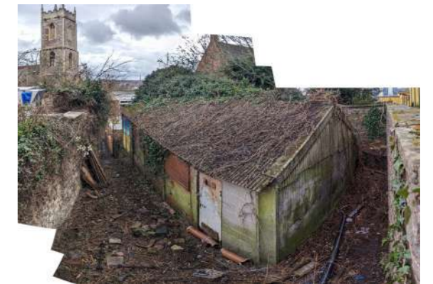
1. Dilapidated scout hut on site
