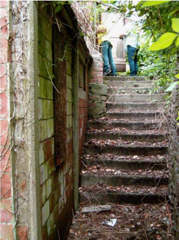
1. Image taken from close to the bottom of the set of steps which runs up the north-eastern side of the scout hut, showing the significant change of level as the result of an upward gradient from south-east to north-west. The structure on the left of the frame is the lower level building, which under the proposed scheme will become in effect an undercroft or 'cellar', and will be used for storage for the new dance/amenity hall. View to north-west.
