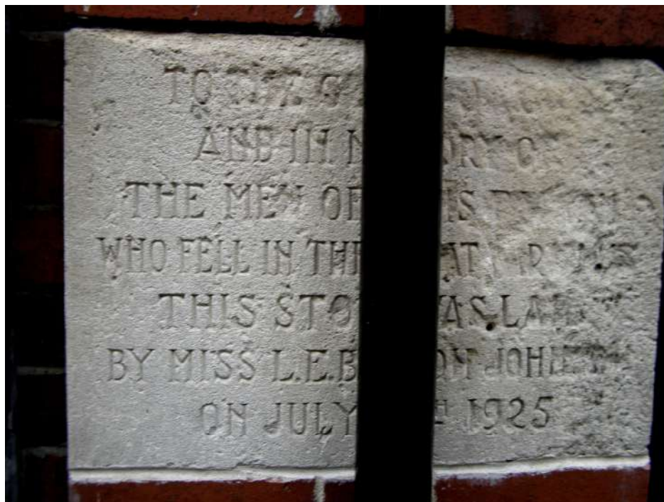
4. The foundation stone of the Memorial Hall, laid in July 1925. Part of the inscription is badly weathered, and it is partially obscured by an unsympathetically placed drain pipe. The stone is located low down at the south-western end of the hall, on its north-western elevation.
