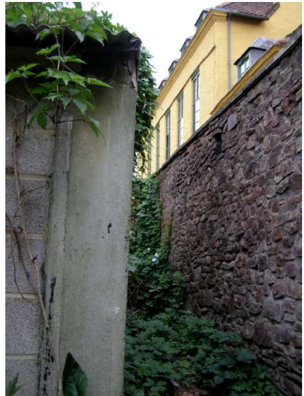
2. Image showing the extreme north corner of the scout hut (left), and the boundary wall between the Manor House and the scout hut/Memorial Hall, showing the upper storey of the Manor House's south-eastern elevation, overlooking the development site. View to west.
