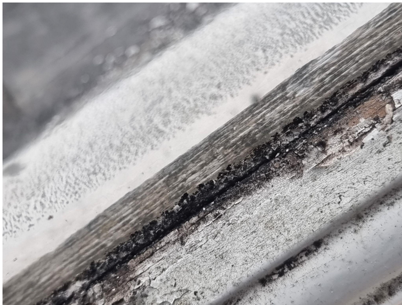
Bare and rotting woodwork internally and externally to the bottom rail where seals and putty have failed.
