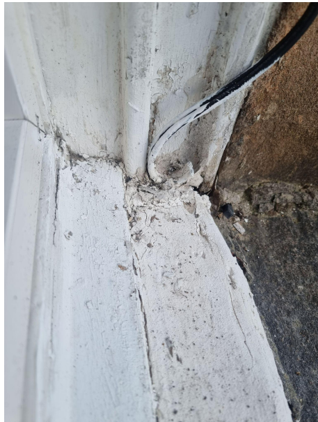
The above photos shows poor repairs to one of the sills on the rear elevation which has been carried out due to rotting and bare woodwork beneath.
