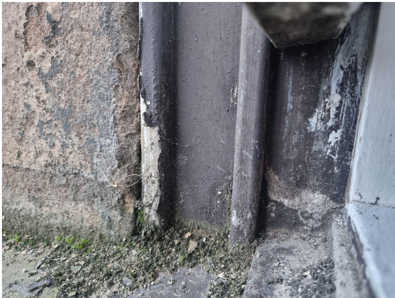
The above photo shows rotting woodwork to the casement and internal pulley pockets.
