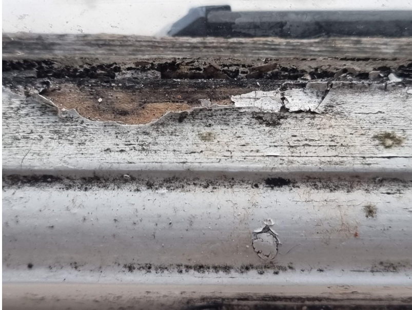
Bare and rotting woodwork internally and externally to the bottom rail where seals and putty have failed.
