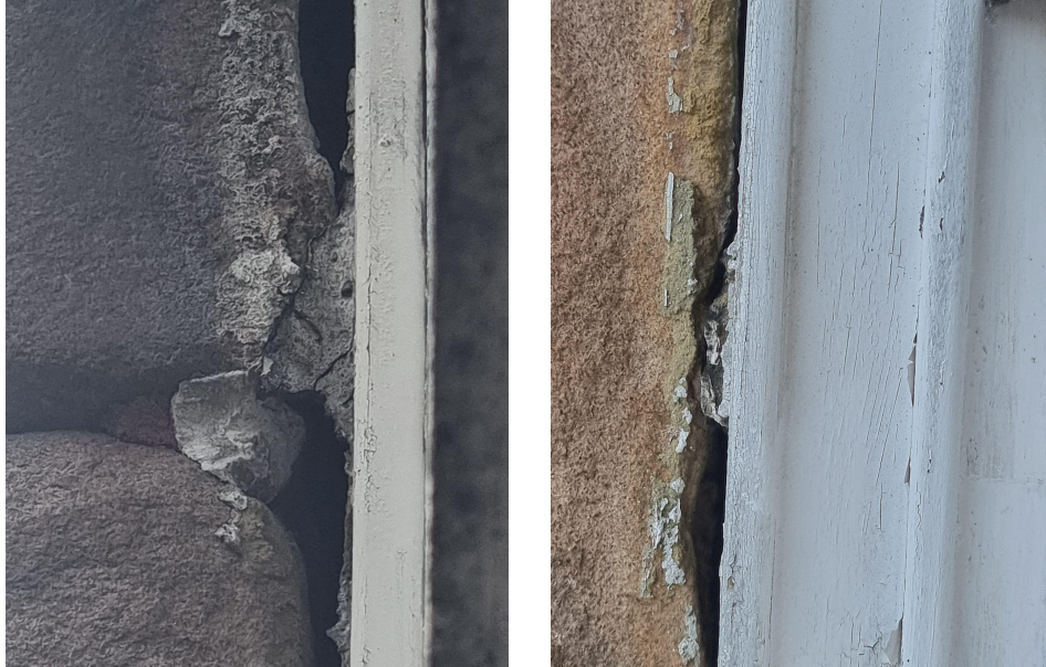
Large gaps around the windows which are allowing water to enter the casement and property.
