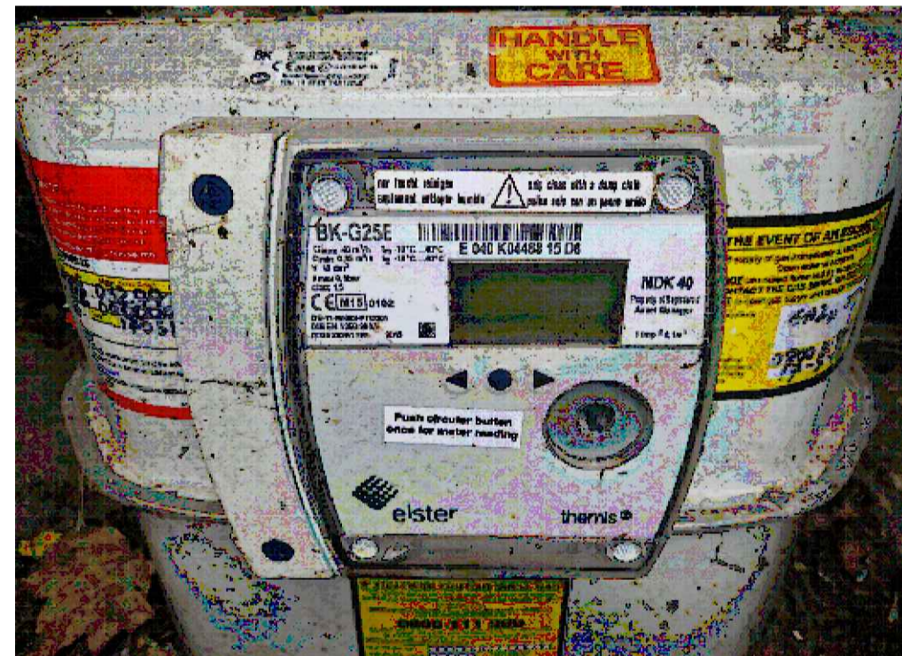
EXISTING GAS METER: METER SIZE/TYPER : BK-G25E (MDK40) METER SERIEL No. : E040 K09468 15 D6 CAPACITY : 40m3/HR DATE : 2015
