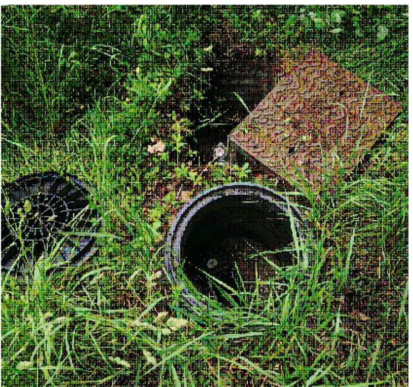
EXISTING MAINS COLD WATER SERVICES (MCWS) METER & STOP-COCK
