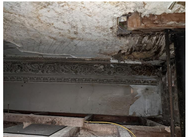
Figure 13: Cornice fragment and damaged lath and plaster ceiling above suspended ceiling
