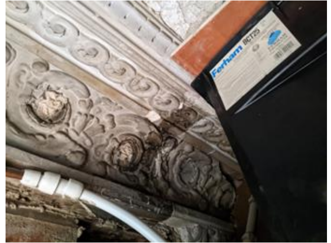
Figure 12: Traces of original cornicing hidden behind the suspended ceiling within the front portion of the flat (above suspended ceiling)
