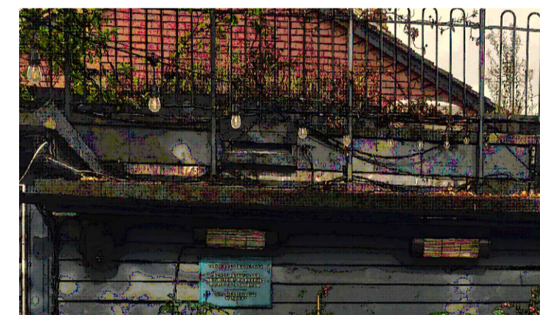
New festoon lighting fixed at high level to building external wall.
