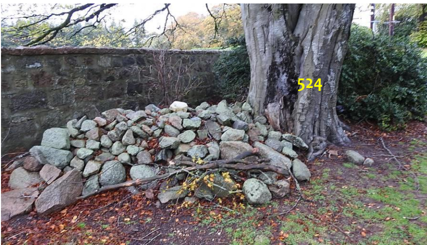
Photo 5: Pile of stones stacked over roots of tree 524, overburdening them. These stones should be removed if they were placed there within the last five years.
