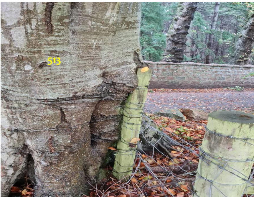
Photo 3: Tree 513 engulfing a fencepost to the south. The tree grows on a retaining wall to the east. It is recommended that the fencepost is removed.
