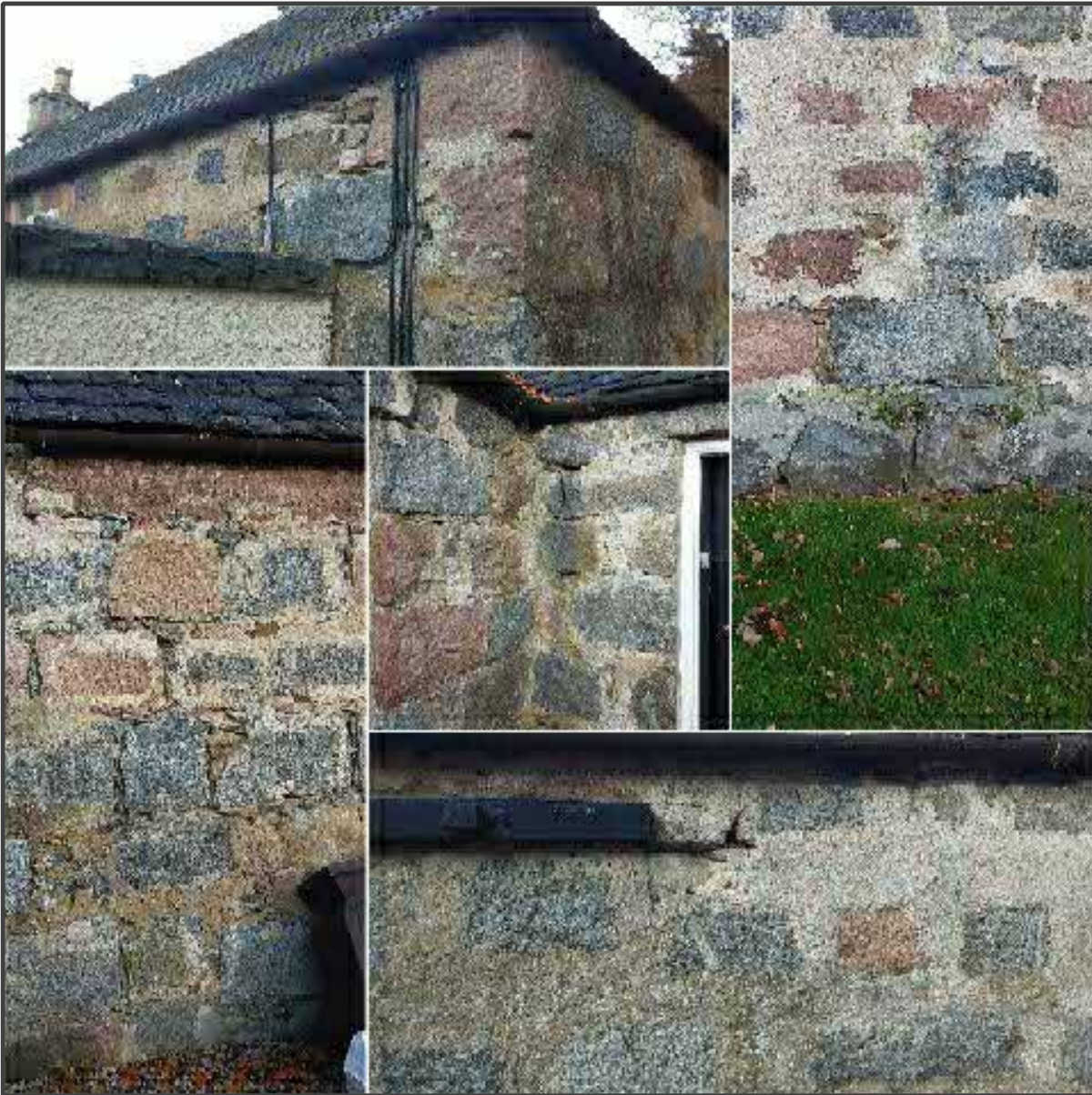
Defective pointing noted to the the external walls.
