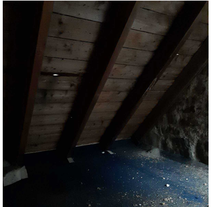
Holes in roof allowing water ingress
