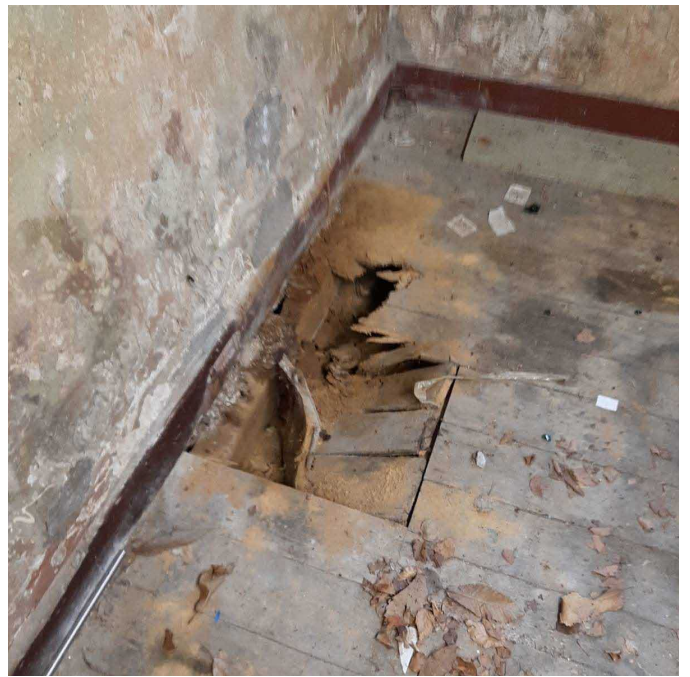
Soft and rotten flooring failed to show timber ground floor joists
