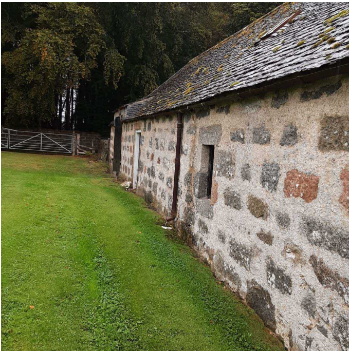
Elevation showing damaged and unconnected drainage
