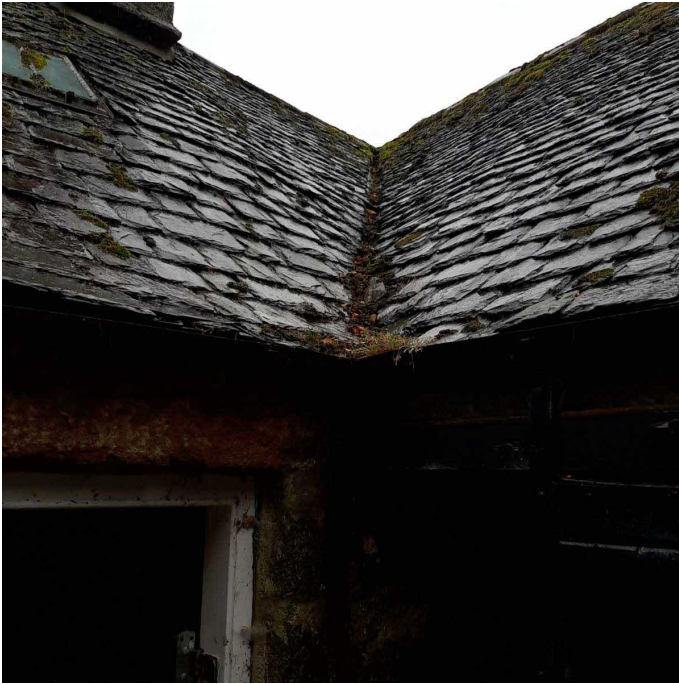
Clogged valley and vegetation on roof
