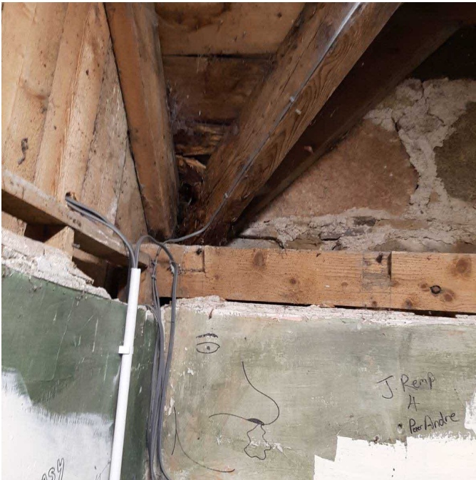
Roof valley showing rotten end
