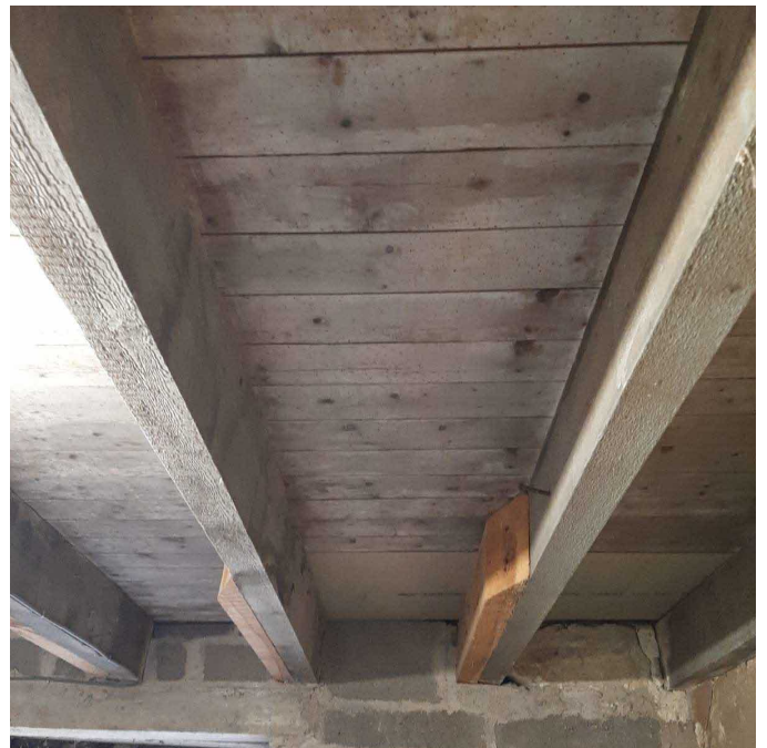
Historically repaired joist ends
