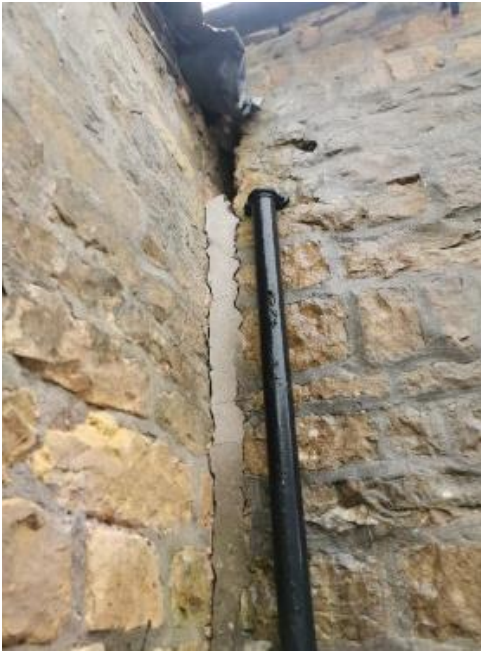
Open Joint Junction Barns 1 & 3
