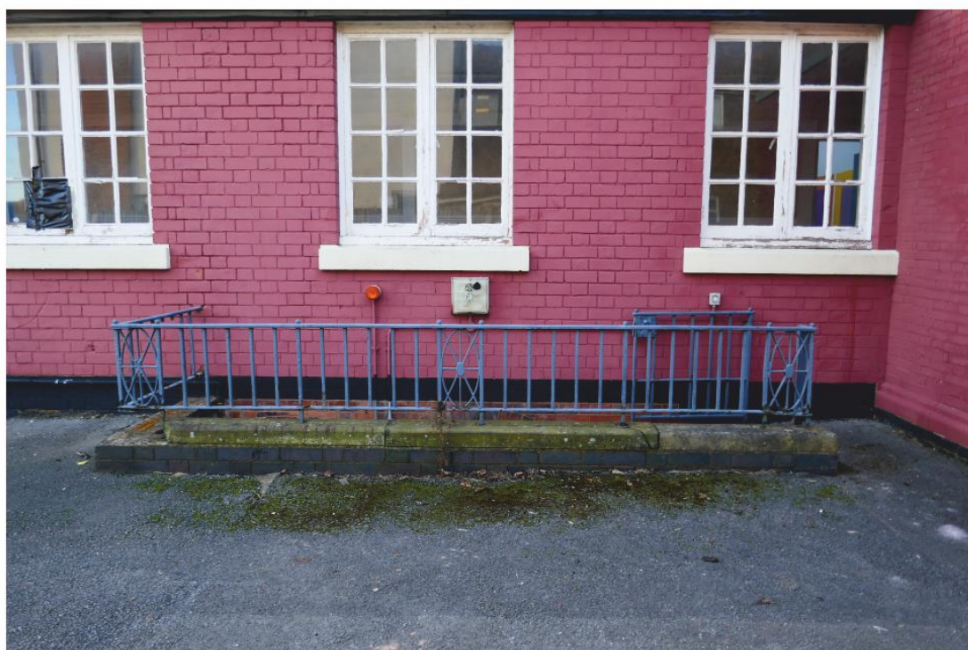
Pl. 24 Metal railings around steps to basement with same decorative motifs as found on the front steps
