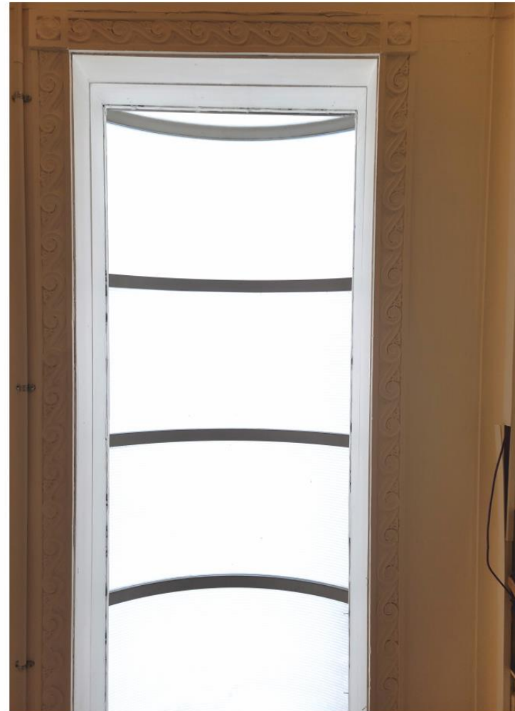
Pl. 30 Corridor ceiling light
