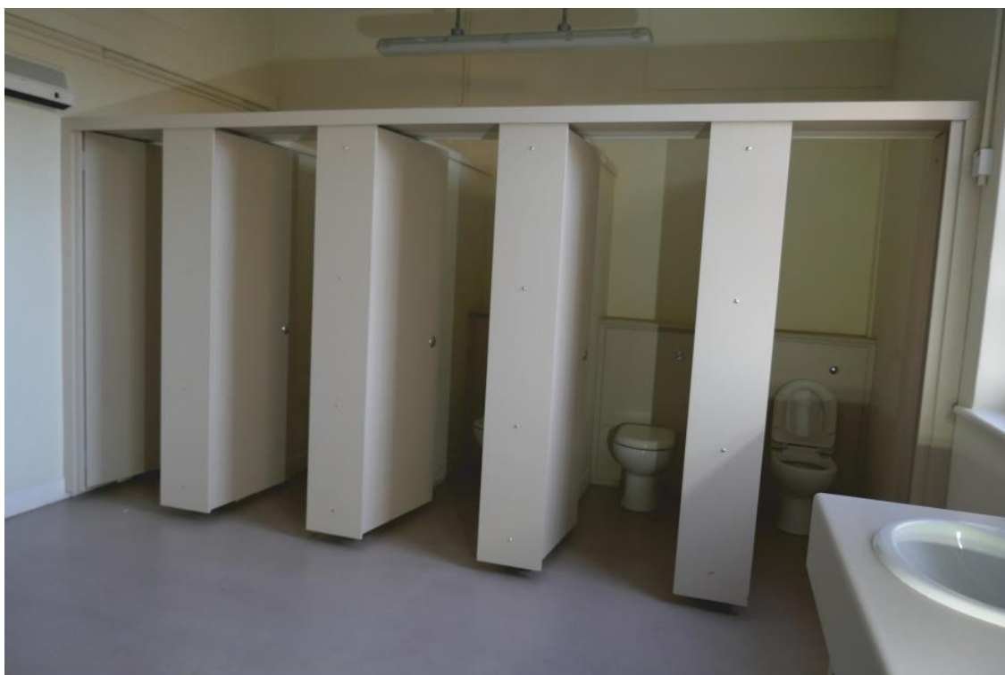
Pl. 63. Ladies' toilet cubicles 9. Blocked side windows just below ceiling
