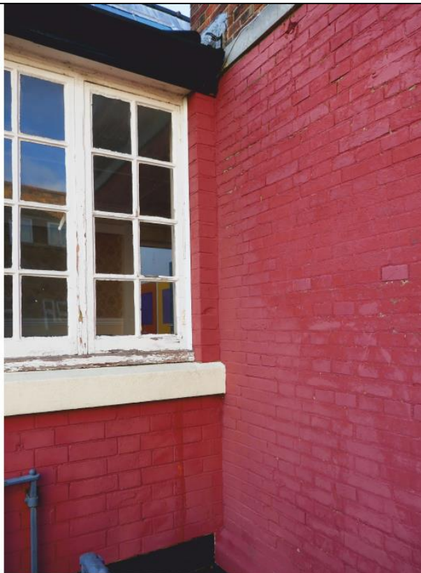
Pl. 23 Detail of the junction between the north and east wing showing the different brick sizes
