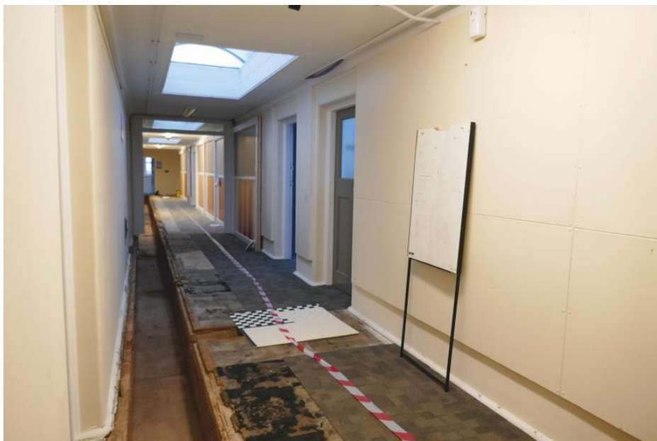
Pl. 33 Conduit running along the north side of the corridor
