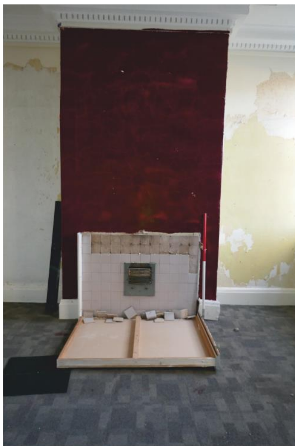
Pl. 57 Room 8 electric fire in chimney breast, hidden behind a plywood panel. ,looking west.
