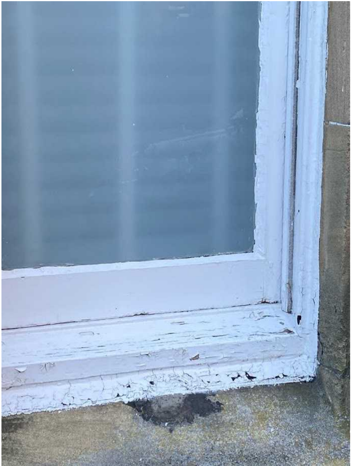
External rotten cills
