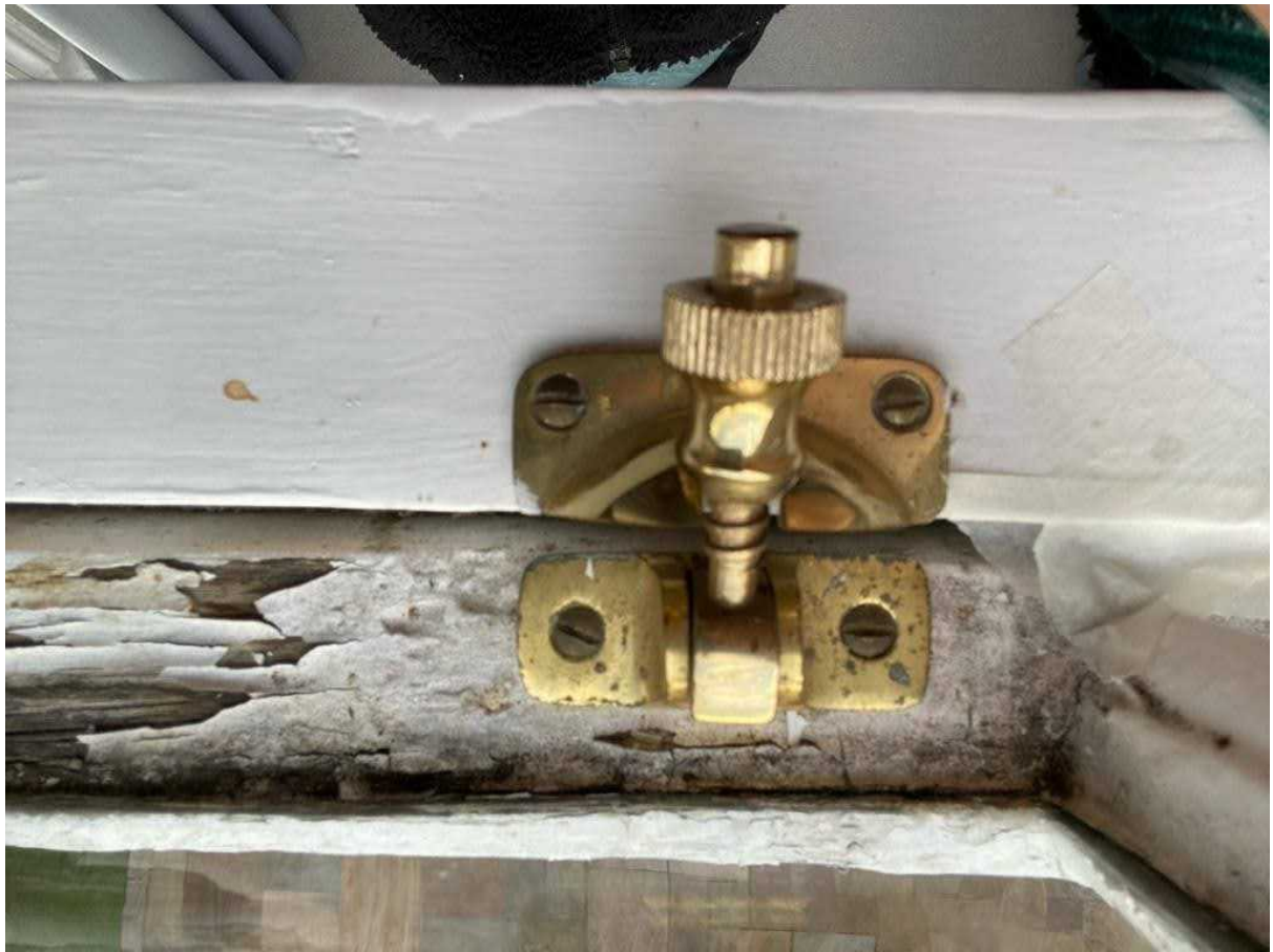
Decay at catches – a security risk
