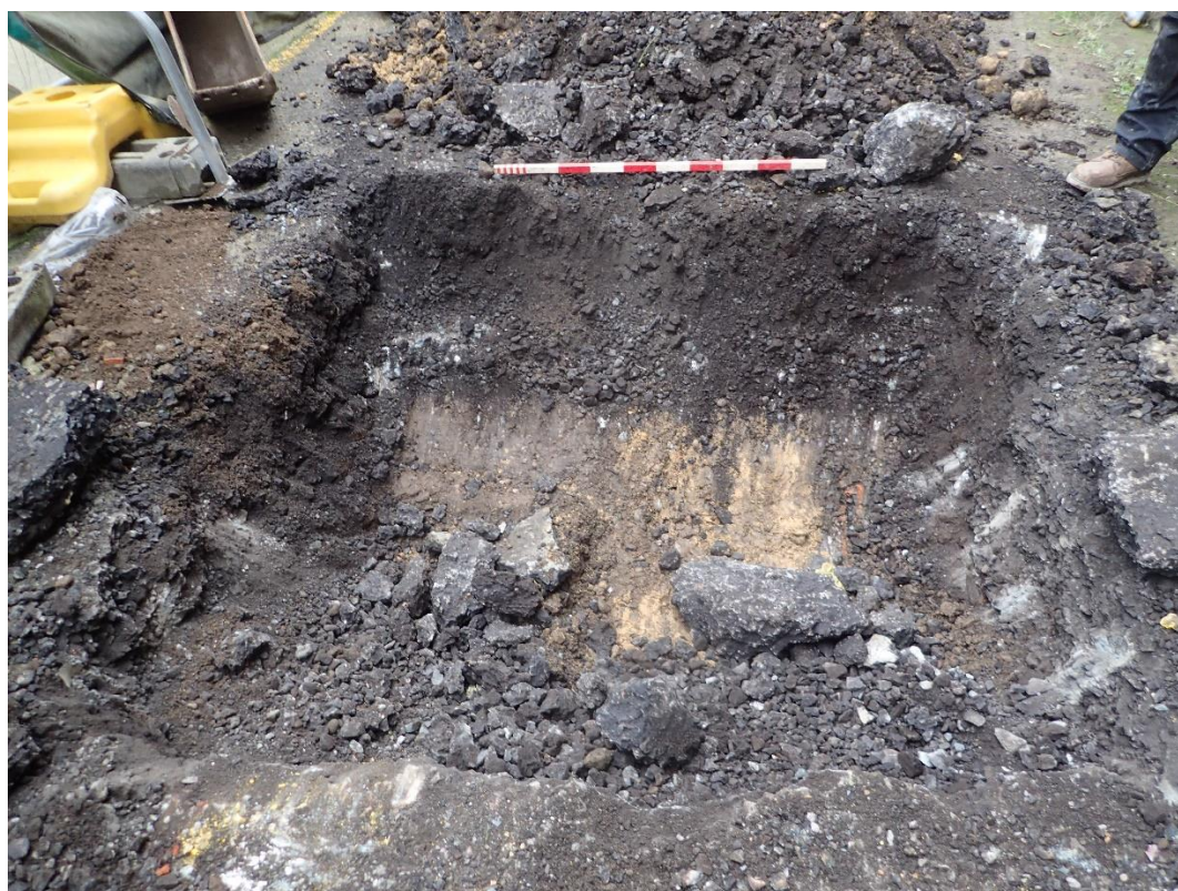
Plate 5: TP2, Section 11, scale 1m, view to south-east. Halted due to live services.
