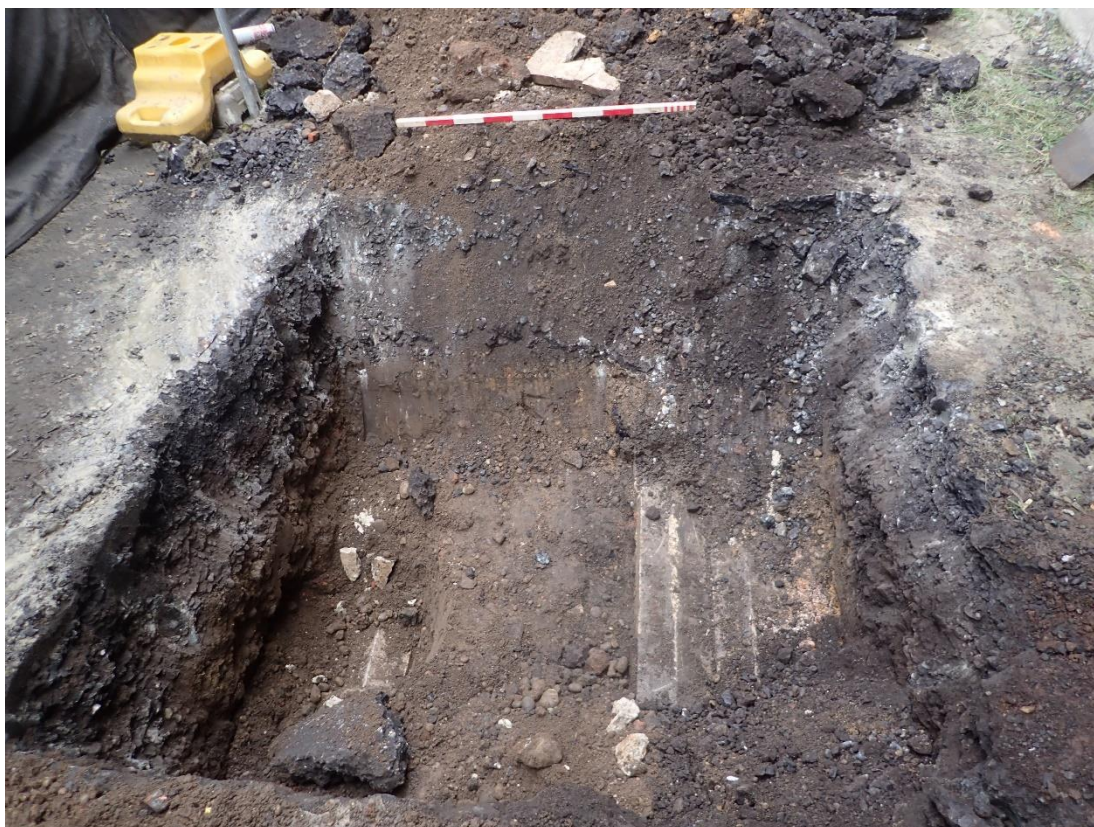
Plate 6: TP3, scale 1m, view to south-east. Halted due to live services. Concrete conduit cap to right of photo.
