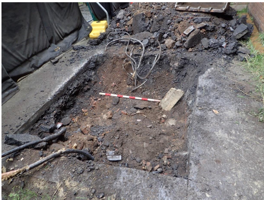
Plate 7: TP4, Section 13, scale 1m, view to south-east. Halted due to live services.
