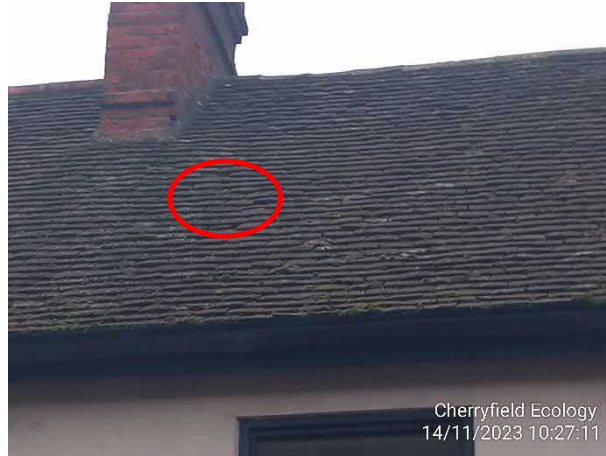
Figure 7: Examples of gaps present in B1
