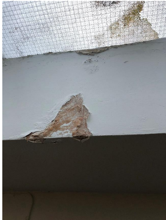
Photograph 2- Spalling plasterwork 1 st Bay
