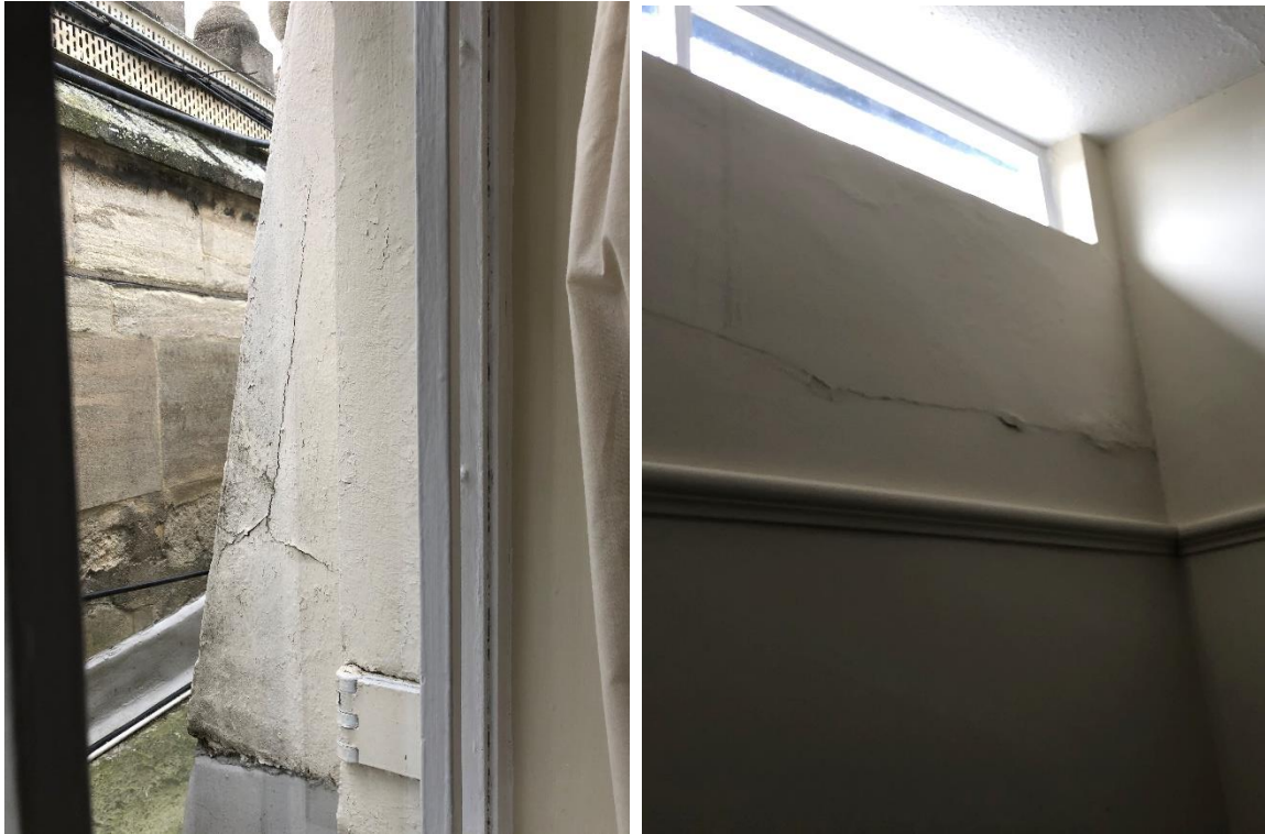
Photograph 8- Cracking to Rendered Finish to RC Column (Room 5) Photograph 9- Horizontal Crack to Perimeter Wall (Room 7b)
