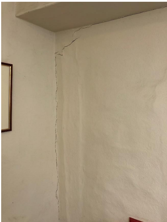
Photograph 11- Cracking in Corner of Half Landing North Stair
