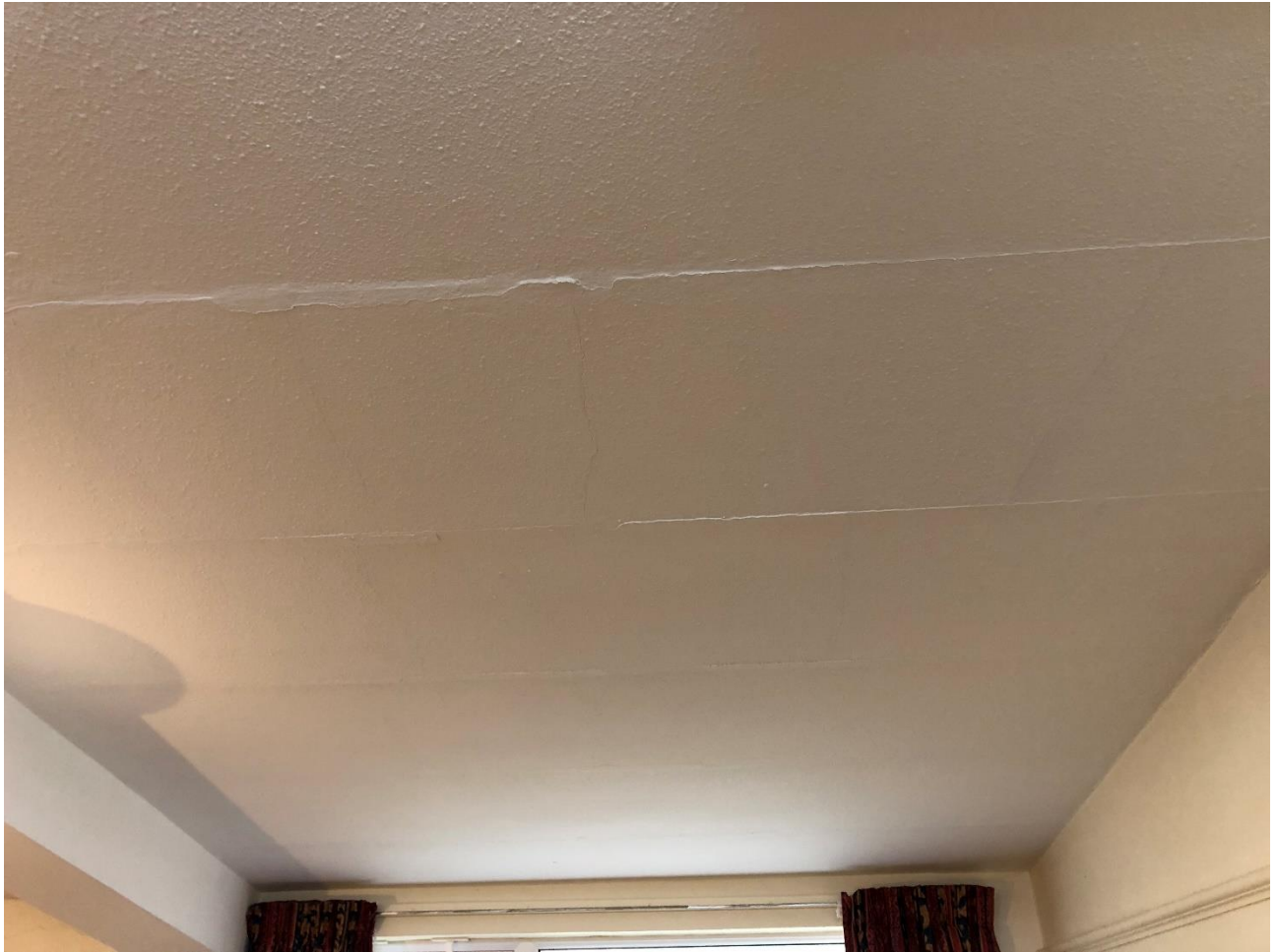
Photograph 5- Typical RAAC Bay Bedroom (Room 3)
