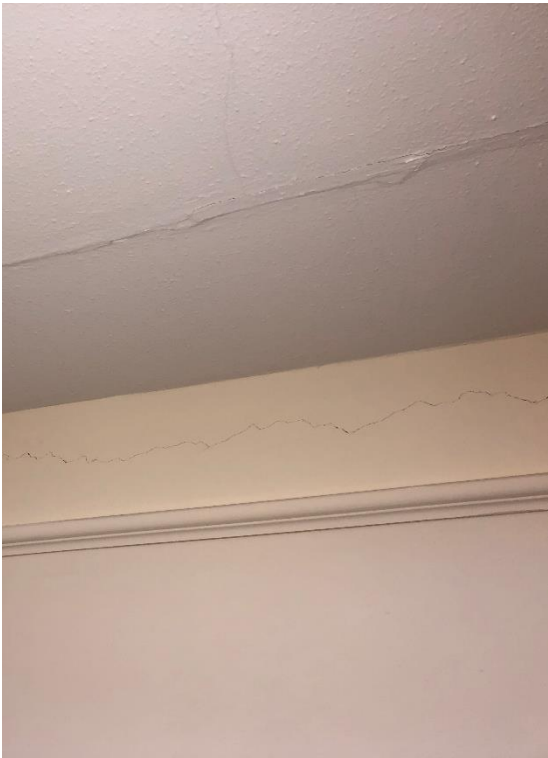
Photograph 6- Horizontal Crack to Perimeter Wall (Room 3)
