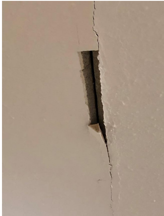
Photograph 7- Failed Joint (Room 3)
