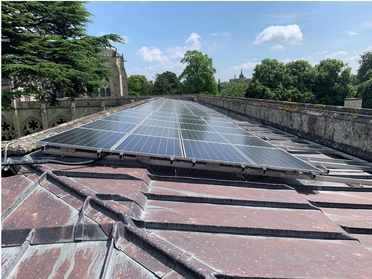
Figure 5: The PV array over the south cloister walk at Salisbury Cathedral. As at Tom Quad, the roof here has a very shallow pitch and features a parapet on its long sides. The PV cells therefore have minimal to no visible ‘footprint’ from any external vantage point – including the Grade I Bishop’s Palace to the east (visible here just to the right of centre) and other listed buildings beyond it along Exeter Street.
